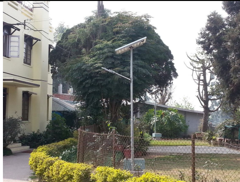
New Solar powered street lighting at Albella
