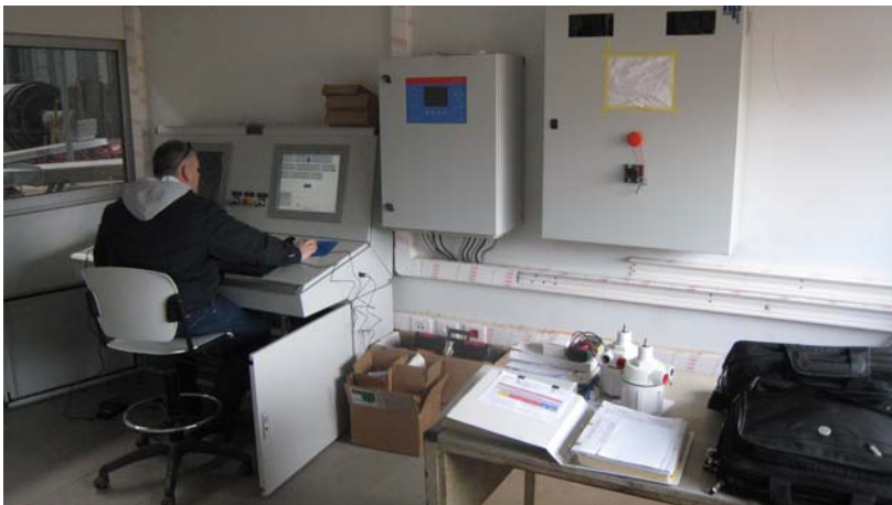
PLANT OPERATOR'S CONTROL ROOM
