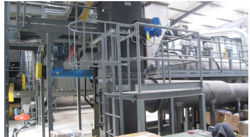
BLACK HEAT FURNACE DELIVERING HEAT INTO TORREFACTION REACTOR
