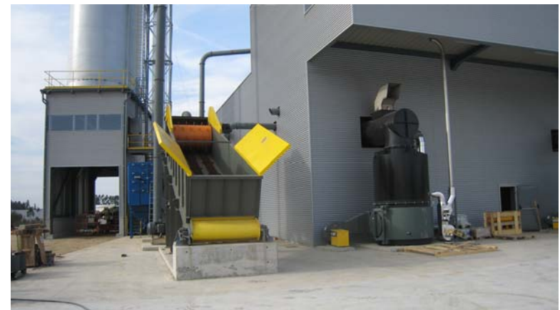
OPEN-TOP, LIVE-BOTTOM HOLDING HOPPER INFEDING RAW BIOMASS INTO PROCESS
