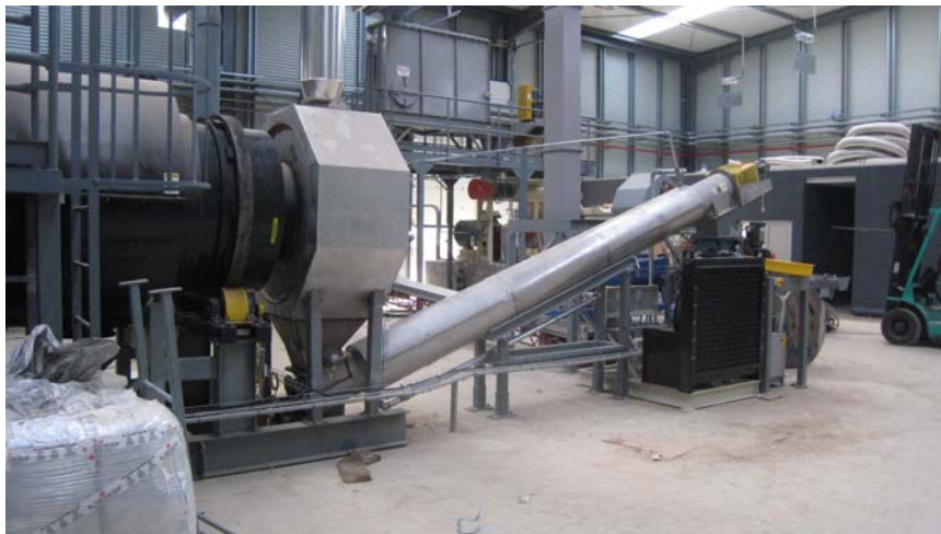
DISCHARGING INTO TORREFIED MATERIALS COOLER
