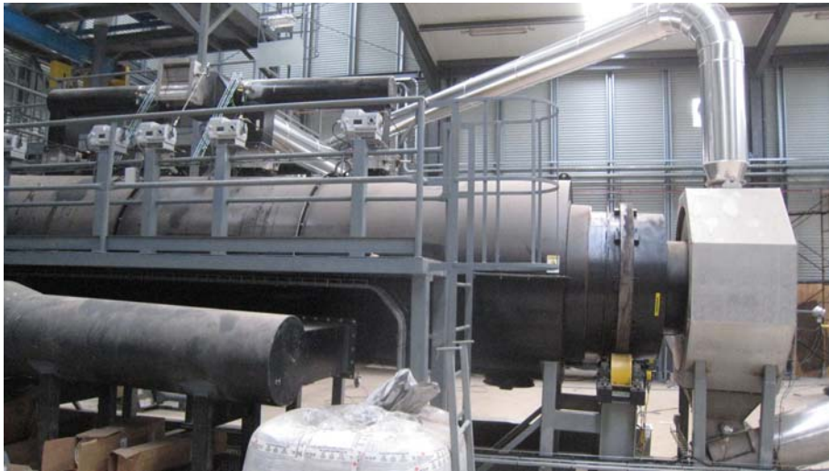
TORREFACTION REACTOR'S VOC & TORREFIED MATERIALS SEPARATOR
