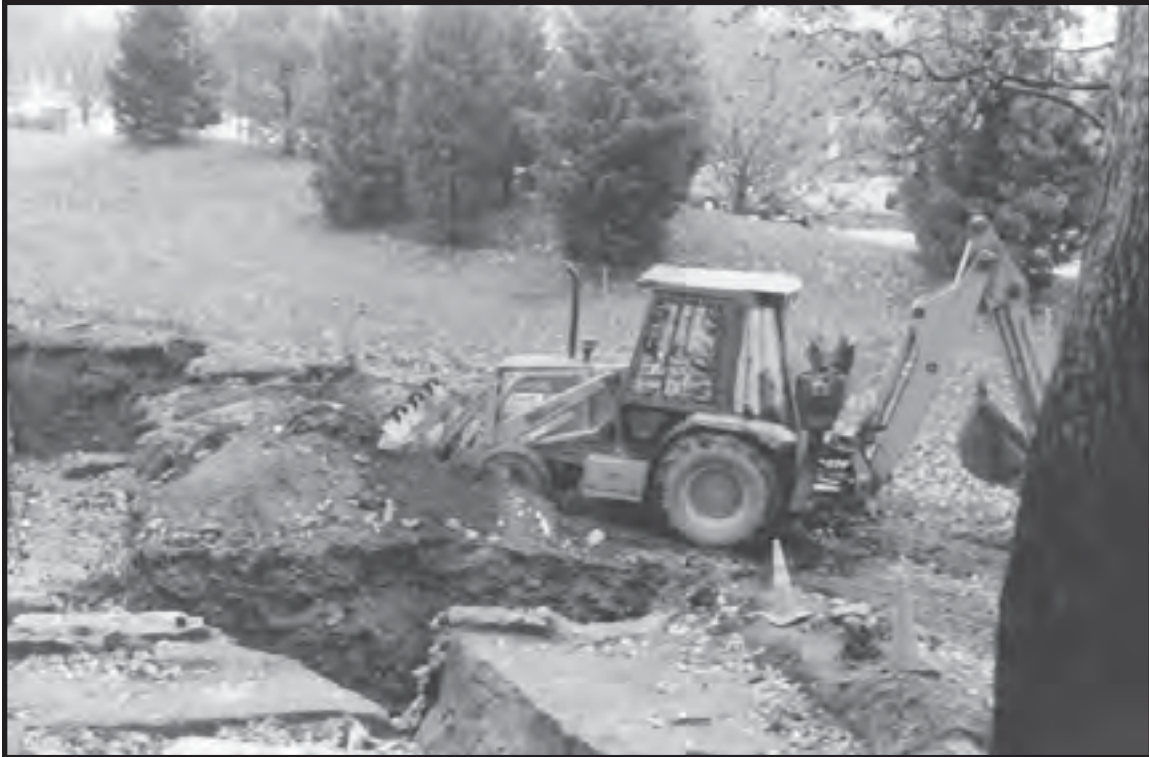
Plate 4.86. Lambert/Douglas Plantation and Rosey Hill Mansion Site: view looking southwest showing mechanical removal of fill from the basement of the Rosey Hill Mansion. North wall of mansion in foreground (Photographer: George Cress, November 1997) [HRI Neg. #97045/10:18].
