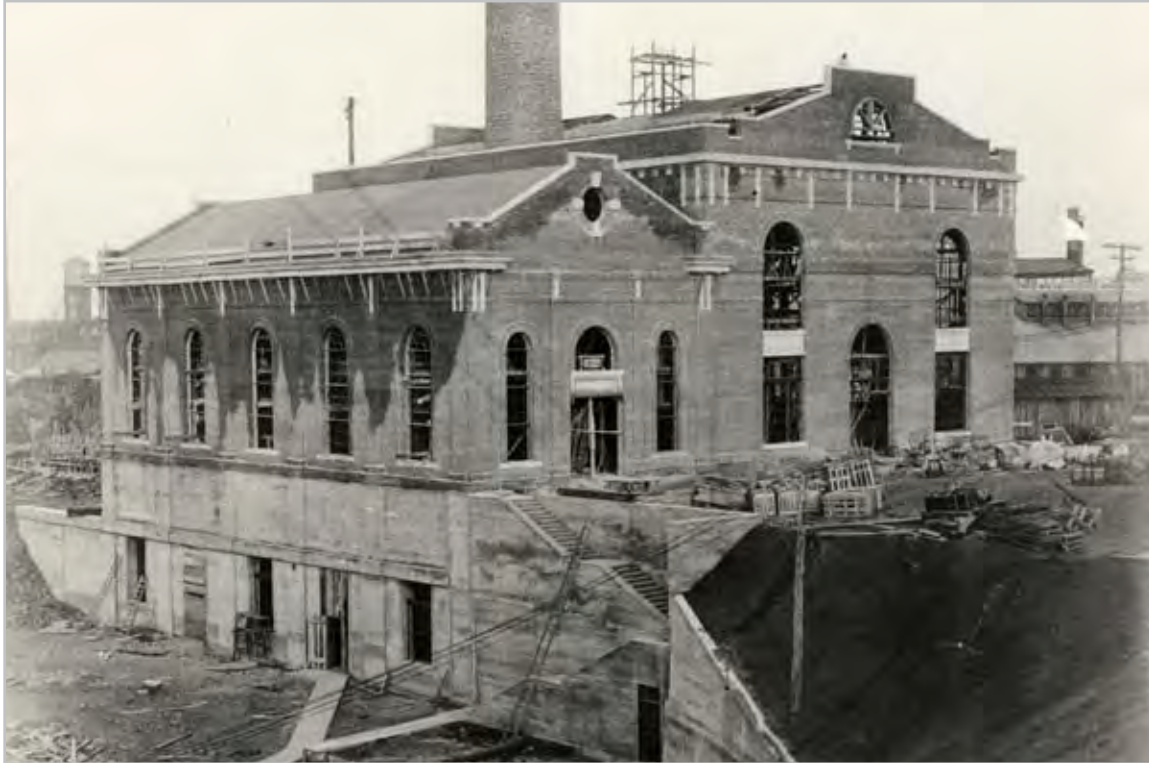
Plate 5.13. The S.U.M. steam plant under construction, looking southeast, circa 1915. The steam plant's primary purpose was to generate electricity in back-up of the hydro-electric plant when water flow in the Passaic was low. It also supplied steam for heating and processing to about a dozen mills, including the Waverly/Mallory mill complex. After the steam plant shut down in 1958, the ATP's Standard boiler house took over as the central steam plant for the district. Source: Paterson Museum Collection.
