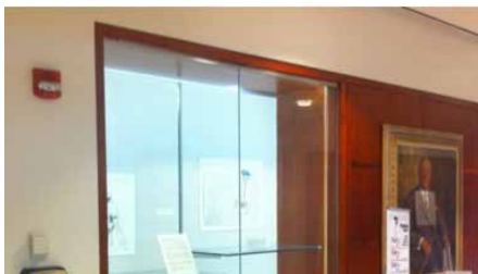
Wall-mounted Alert Beacons are installed in strategic locations throughout the Washington University in St. Louis campus.
