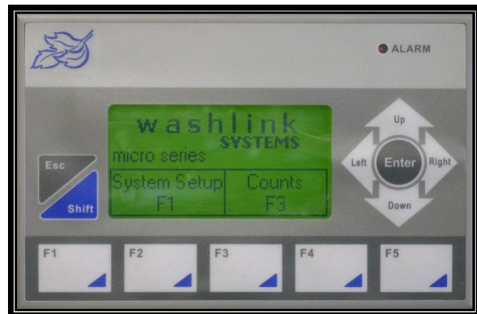
Adjust “on the fly” (no shutting down car wash for system changes)
