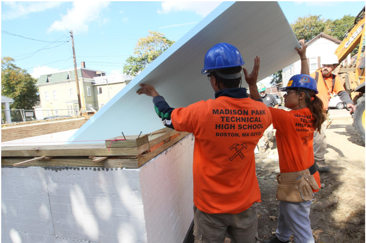
JOANNE RATHE/GLOBE STAFF Carpentry students from Madison Park Technical Vocational High School are helping to build a home at North Avenue in Roxbury.
