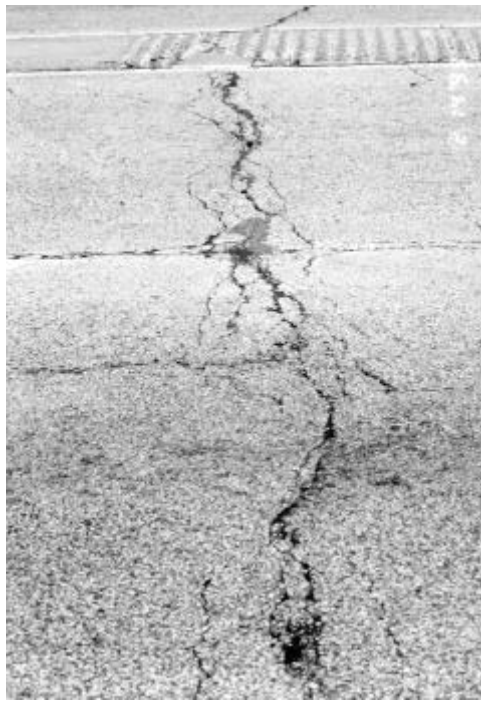
Figure 3. Pavement candidate for crack repair.
