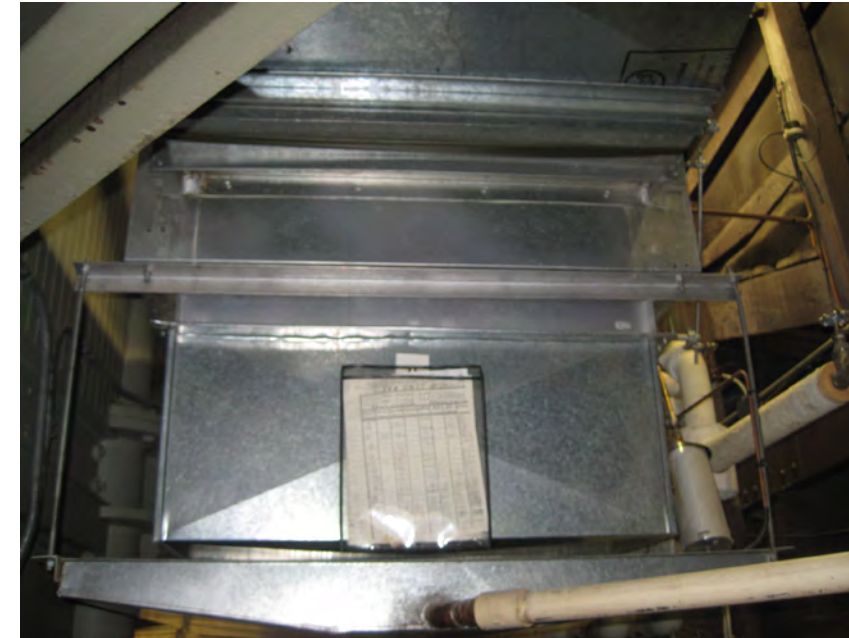
Figure N.02.01 - Existing Attic Air Handling Unit
