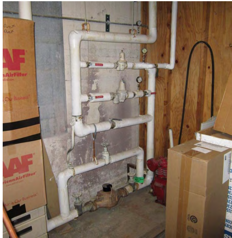
Figure N.02.02 - Existing Capitol Bldg Water Service Branch with Meter & Pressure Reducing Station
