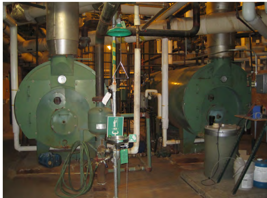
Figure N.01.04 - Existing Herschler Boilers
