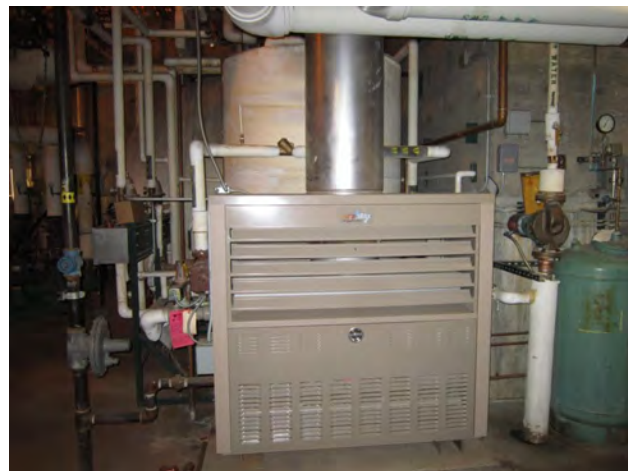
Figure N.01.09 - Existing Gas-Fired Domestic Hot Water Heater, Herschler Basement MER
