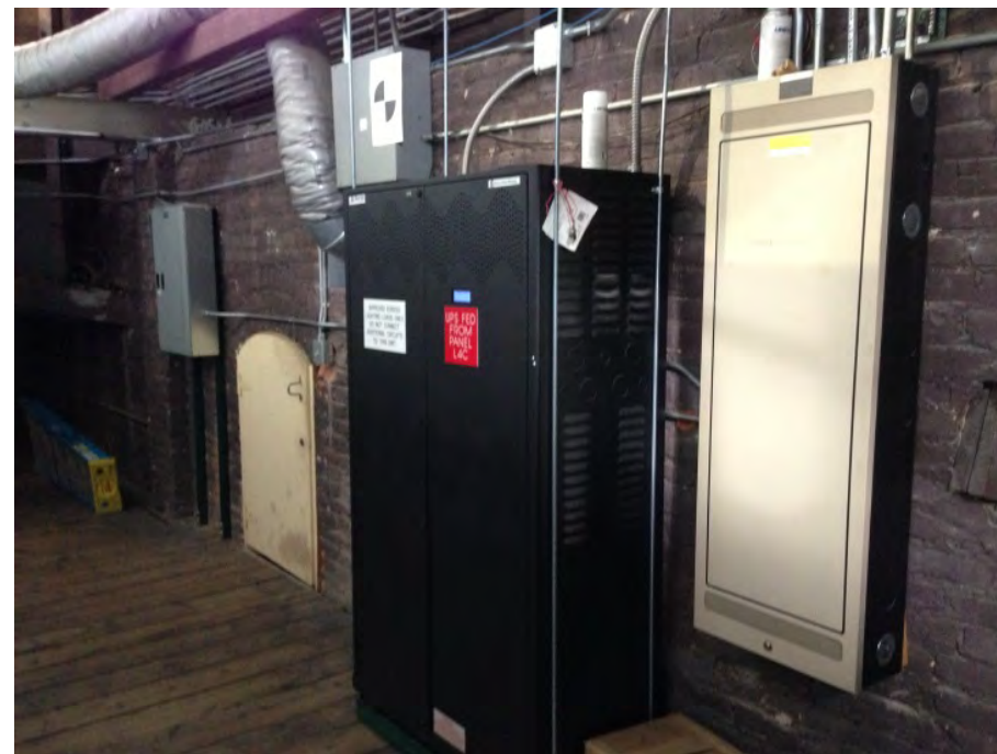
Figure N.02.07 - Existing Emergency Lighting UPS System (Attic)
