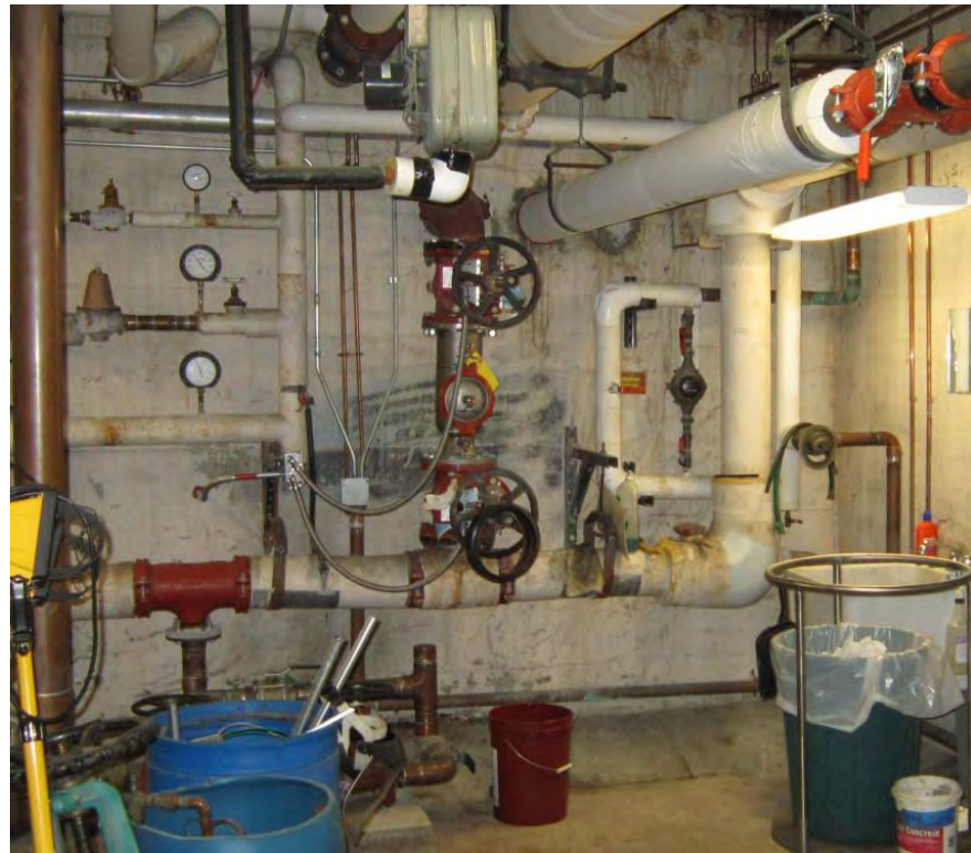
Figure N.01.06 - Existing 6” Domestic Water Service, BFP & Pressure Reducing Station, Underground Connector Bldg
