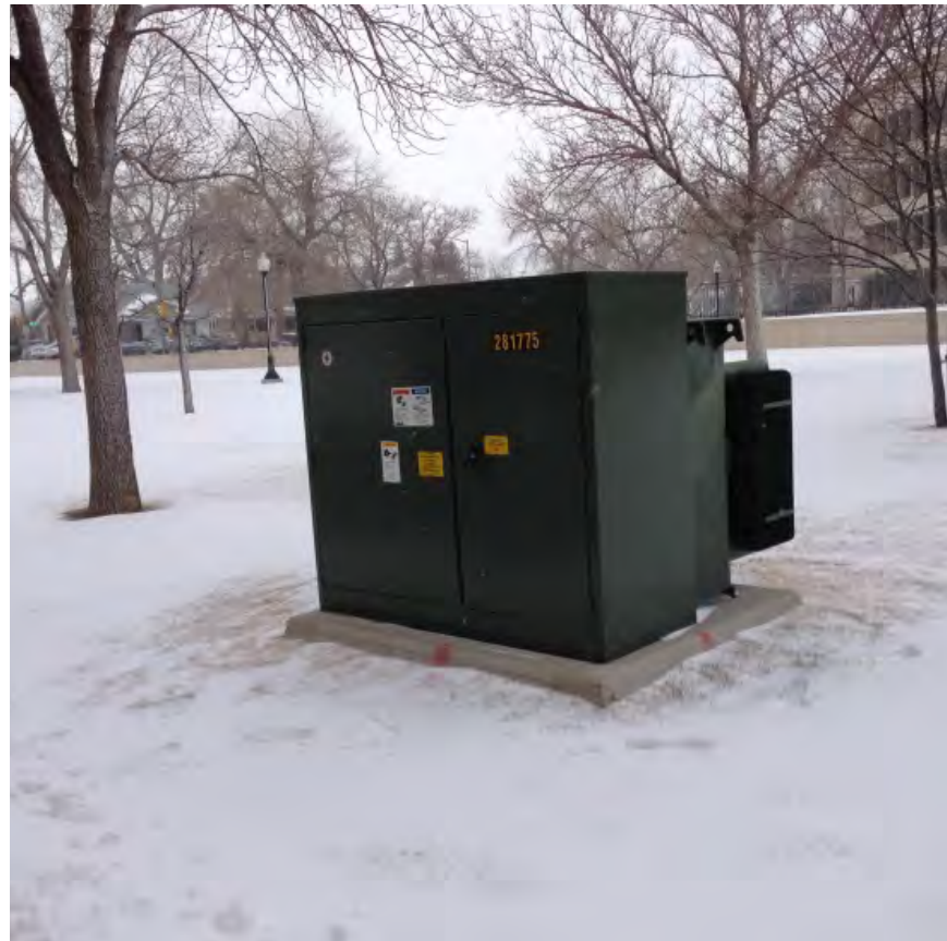
Figure N.01.12 - Existing Capitol Bldg Utility Transformer
