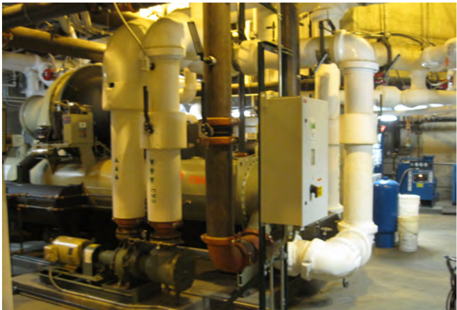
Figure N.01.02 - Existing Herschler Chiller
