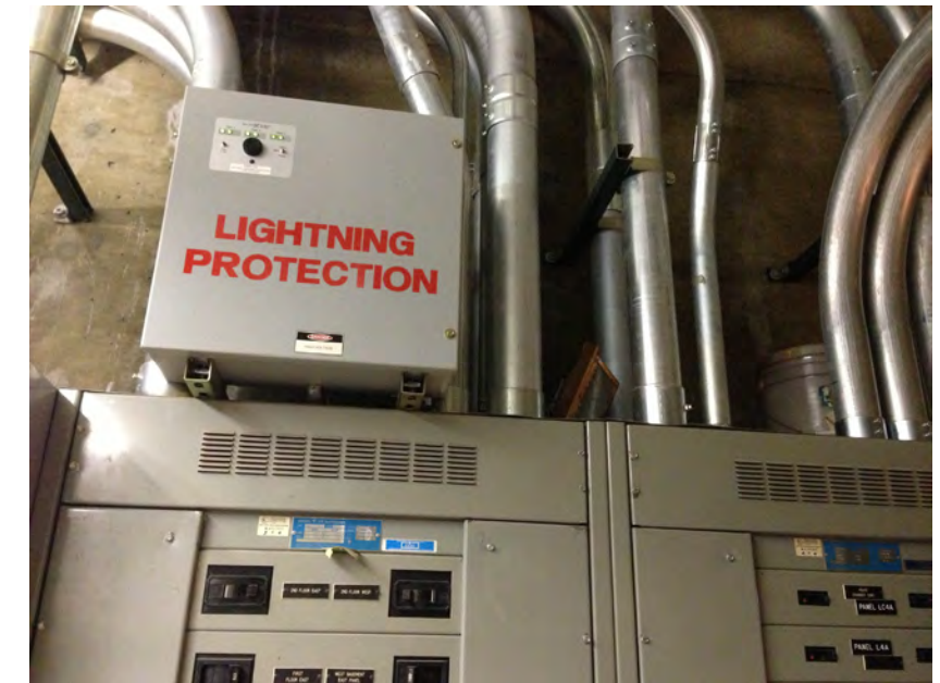
Figure N.02.06 - Capitol Bldg Switchboard Surge Protector, Connector Bldg
