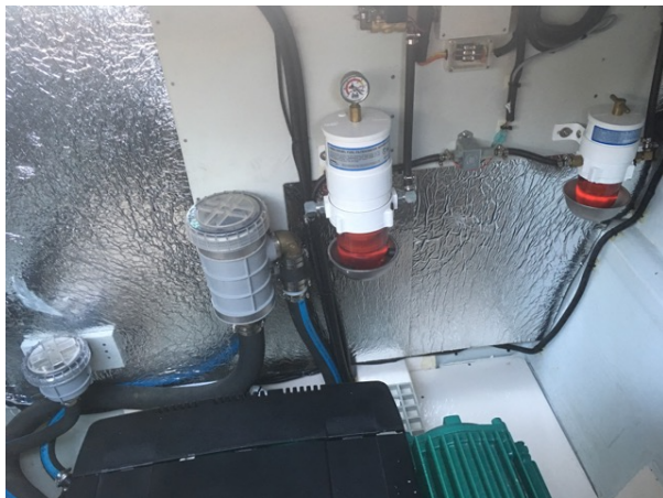
STBD Engine Compartment: Generator and Engine Strainers. Racor filters for Engine and Generator
