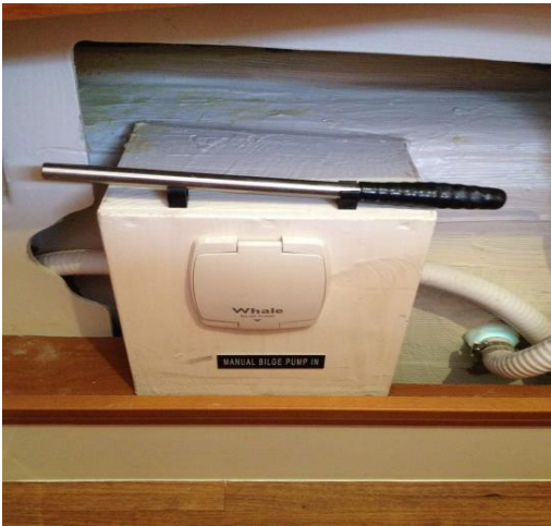
Located in Master cabin STBD cabinet
