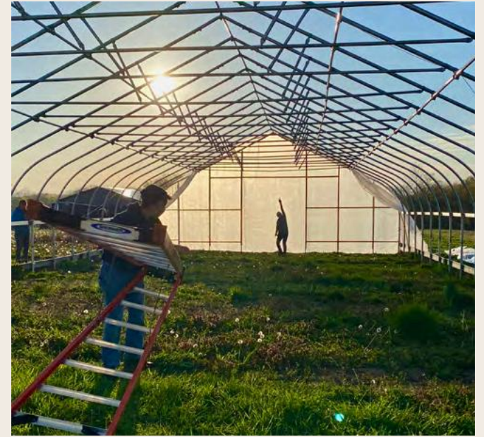
Agraria staff and volunteers, led by VISTA Xinyuan Shi, installed a new high tunnel on Huston Road.
