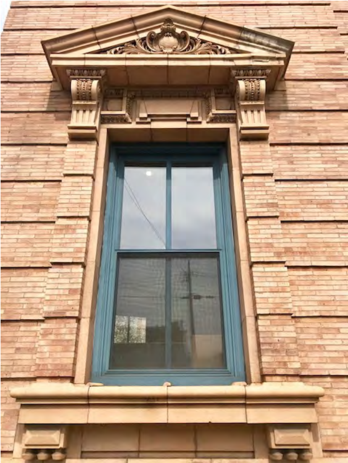
Photo. 6. Former Pennsylvania National Bank Building, Butler St. Façade, Tympanum Window Detail , August 2019. Source: Matthew W.C. Falcone.
