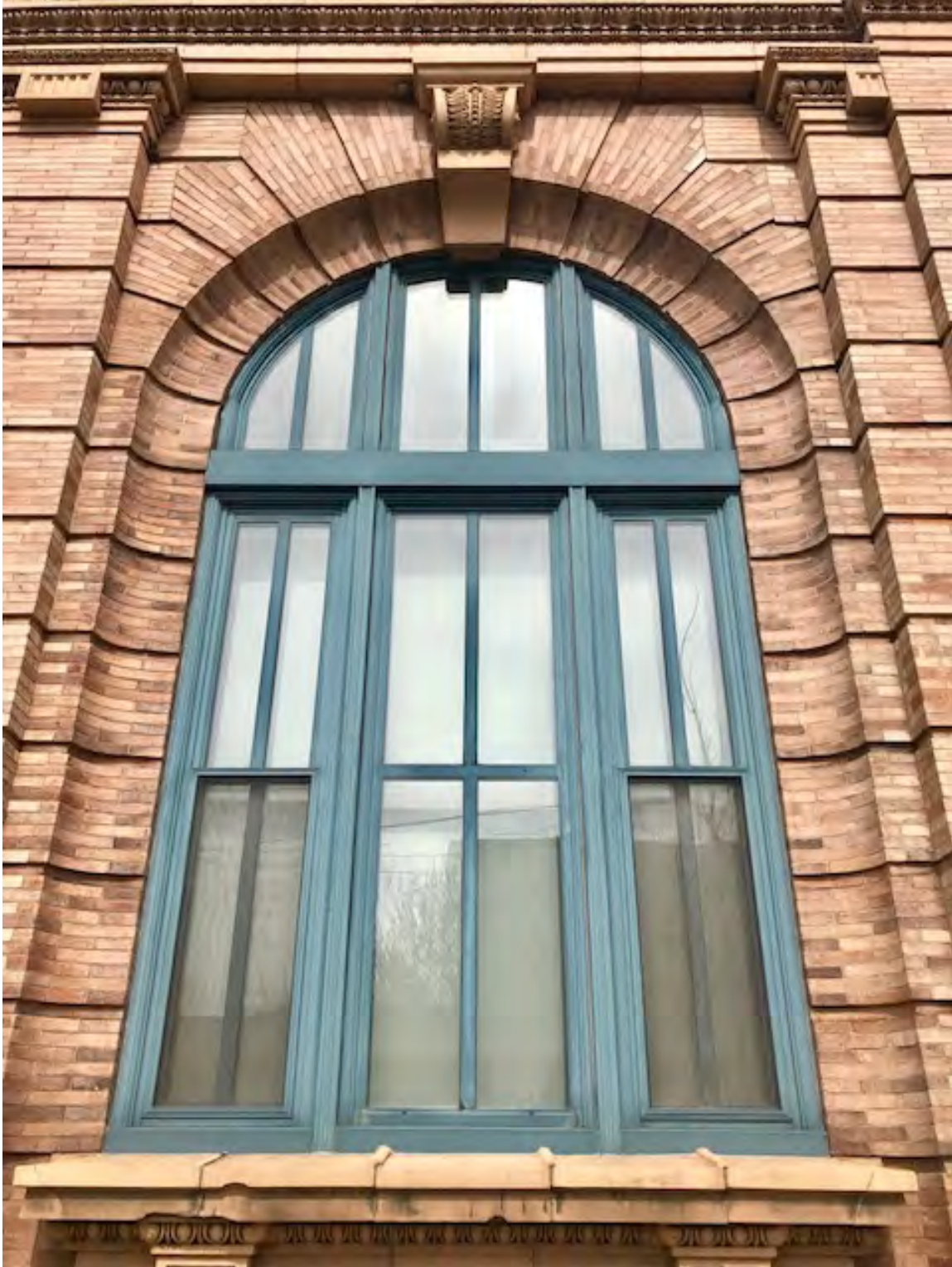
Photo. 7. Former Pennsylvania National Bank Building, Butler St. Façade, Arched Window Detail , August 2019. Source: Matthew W.C. Falcone.
