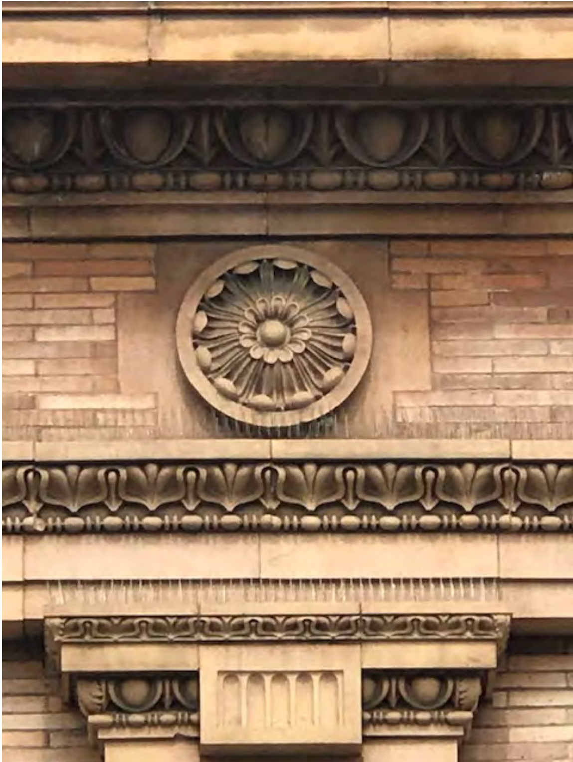
Photo. 8. Former Pennsylvania National Bank Building, Cornice Detail, Terracotta Medallion, August 2019. Source: Matthew W.C. Falcone.
