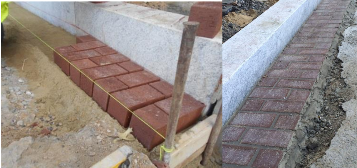
Examples of new granite curb and brick gutter installation this week at Sta 14+50 Georgia Avenue
