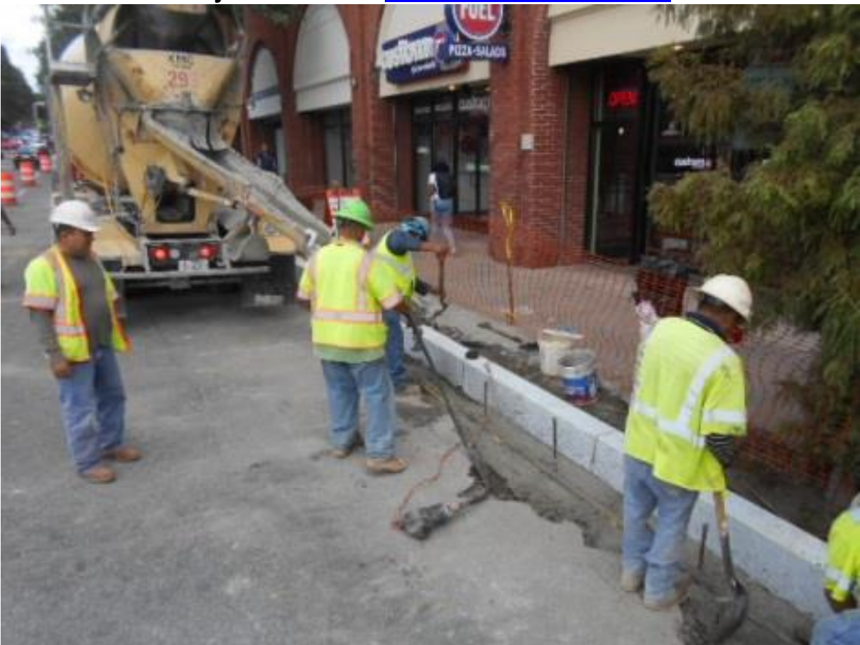
Placement of PCC dry mix for brick gutter foundation at Sta. 14+00 – August 26, 2015
