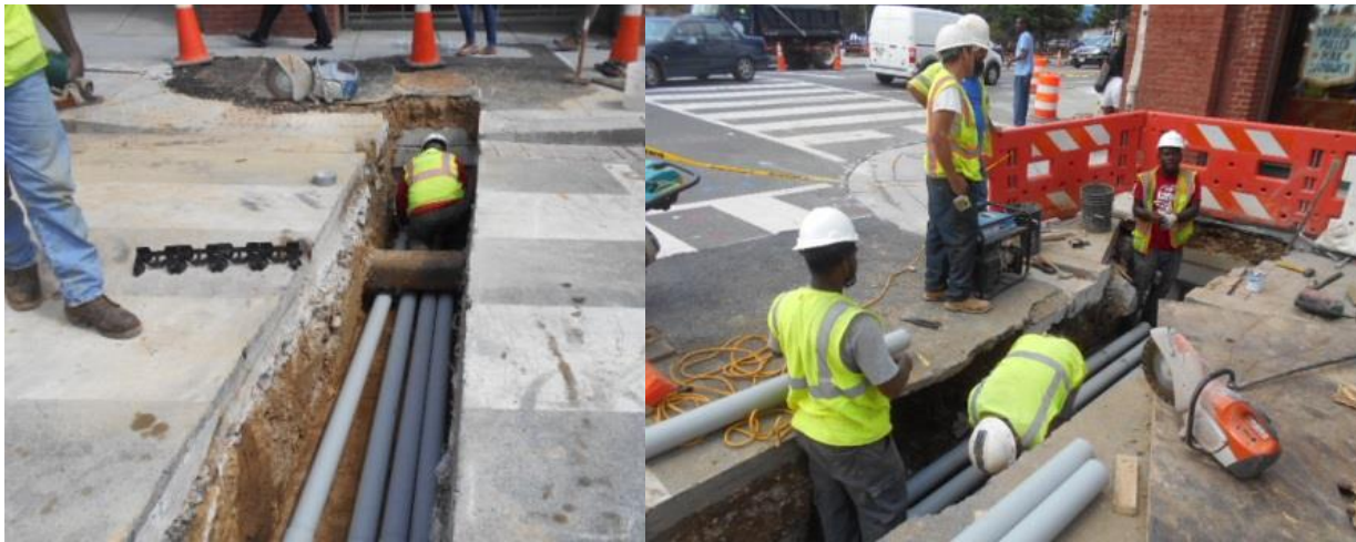
Installation of new PVC conduit at electrical manholes C1 (left) and D2 (right)
