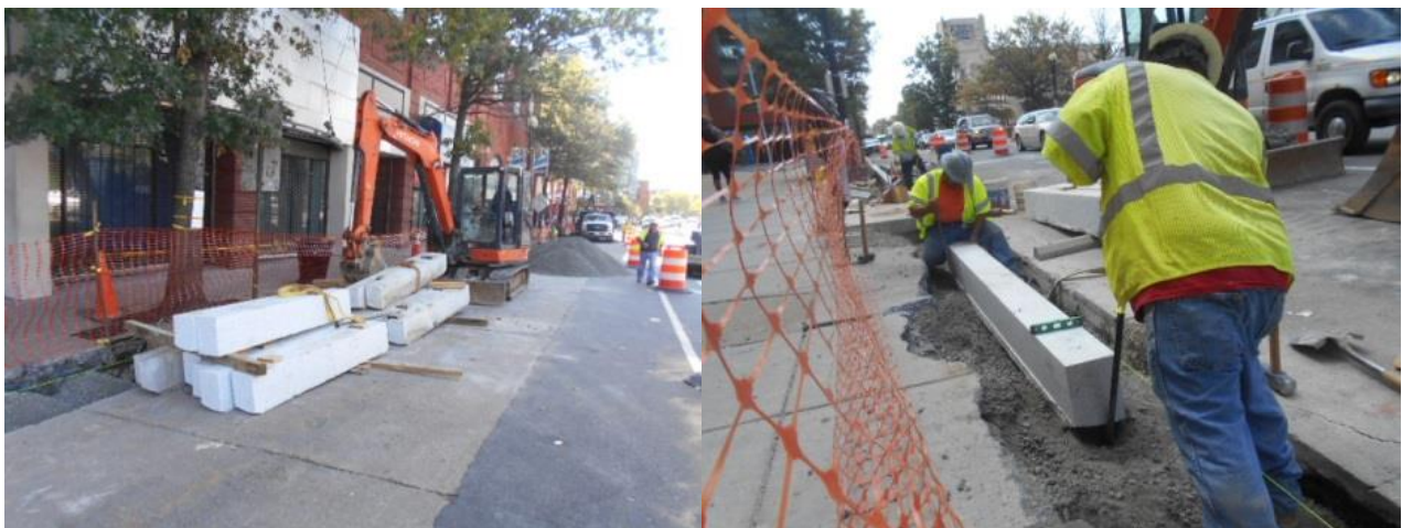
Delivery of new granite curb to site on 8/25/15 and installation of new curb on east side of Georgia Avenue
