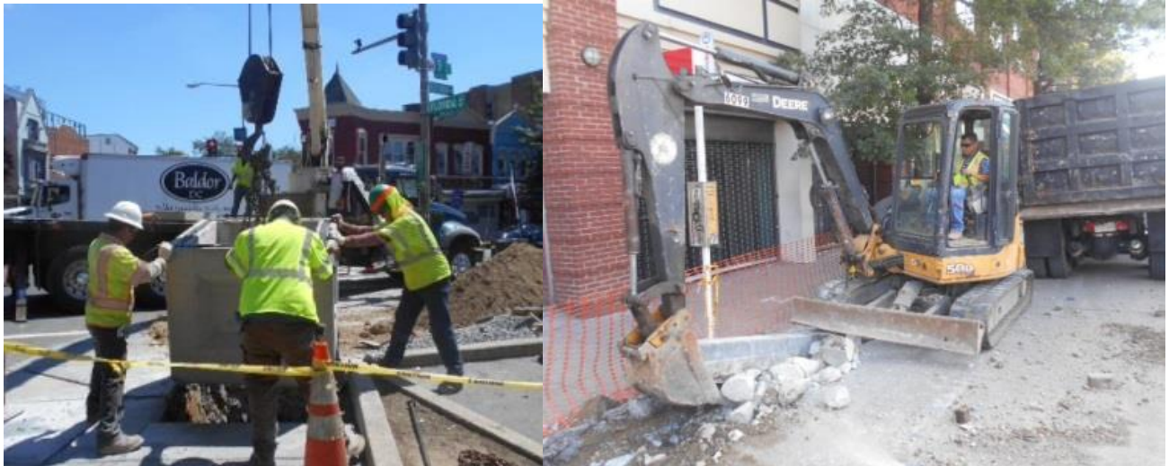
Installation of electrical manhole B5 on 8/22/15, and removal of existing curb and gutter on Georgia Ave
