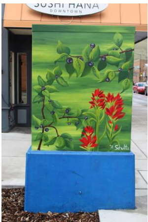
Huckleberry Haven Hannah Schultz Fall 2018 Higgins & Pine Paint
