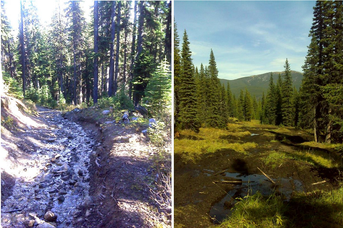
Plate 3. Two photographic examples of ORV trails with deep ruts and erosion from water ponding and drainage.
