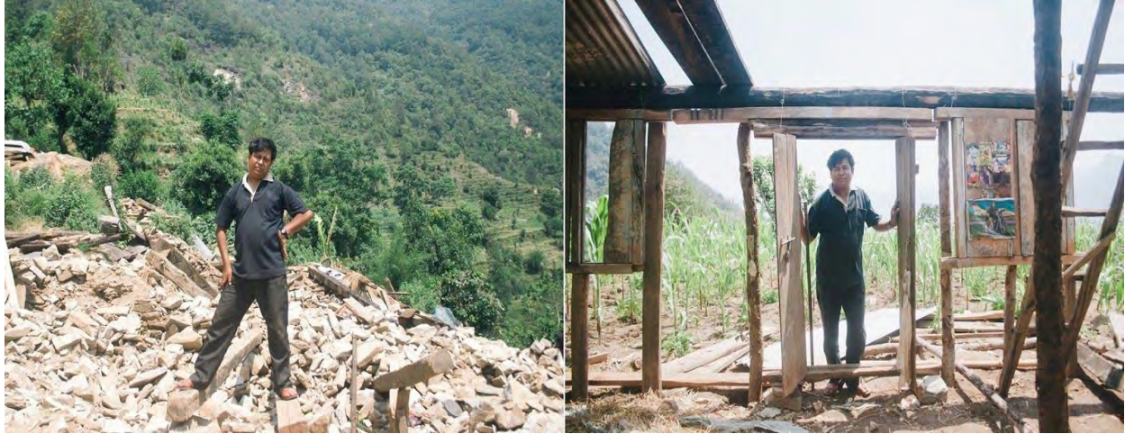
Thulo Kancha Sunwar-34, a farmer from Chittre, Ki-Wool - 5, Sindupalchowk is rebuilding his house by implementing techniques learned from the model transitional shelter.
