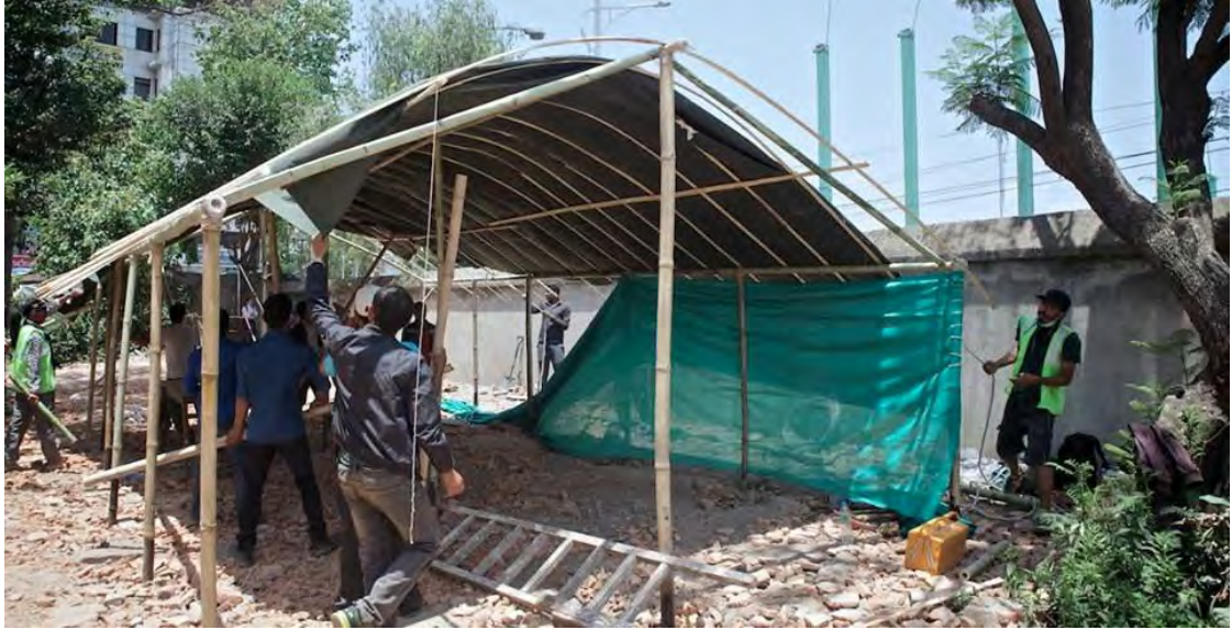
Training local youths on how to make a vaulted shelter in Kathmandu
