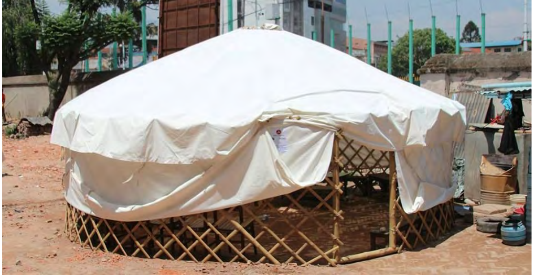
We installed child-friendly Yurts at Durbar High School to serve as Temporary Learning Centres
