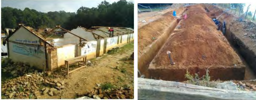
(Left: Remains of the destroyed Shree Narayansthan Higher Secondary School Right: Laying the foundation for the school)
