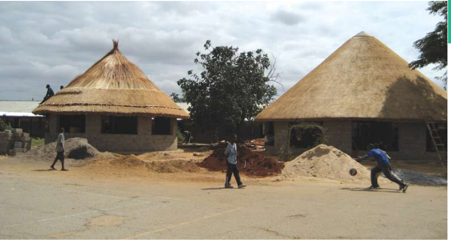
The Reading Room of the first Lubuto Library under construction in February.
