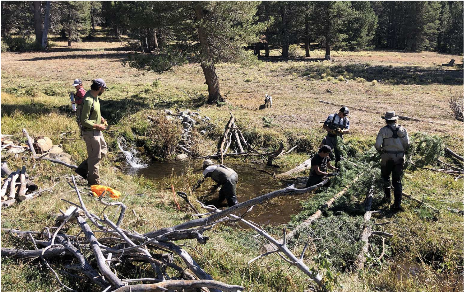
Field crew installing low-tech structures at Casa Vieja pilot project in 2021. Photo courtesy Nick Bouwes.
