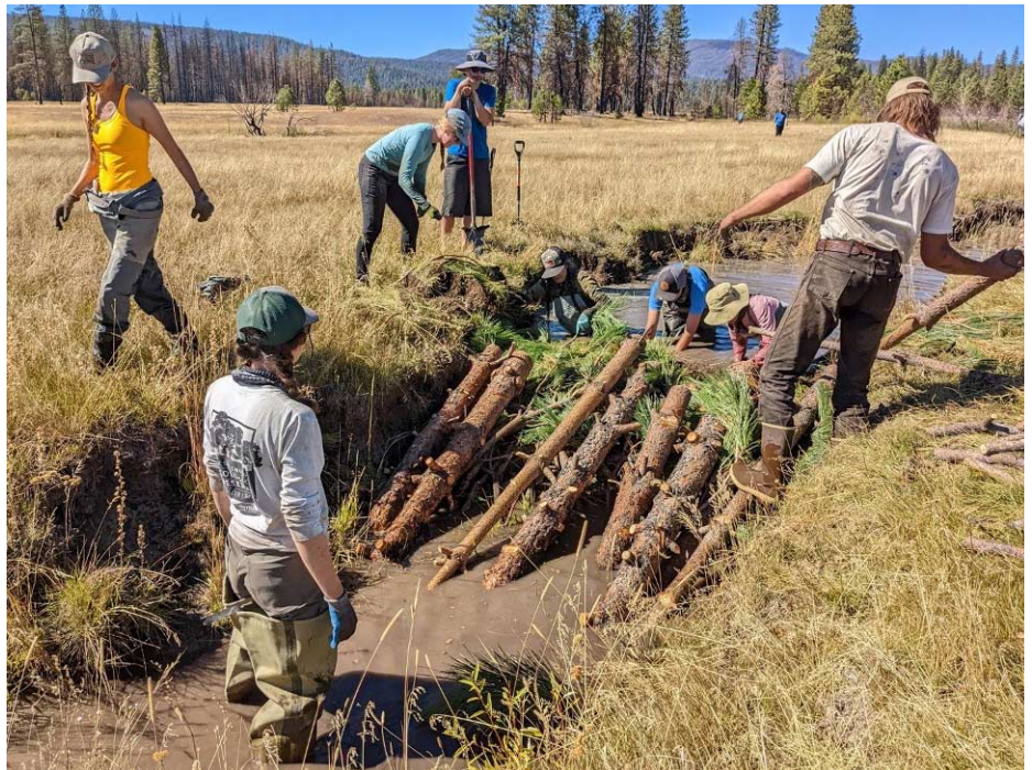
Participants of the Fall 2022 “Build Like a Beaver” training led by members of the Cal PBR Network build instream structures to mimic beaver in Yellow Creek. The training was held on two adjacent Plumas County properties stewarded by the Maidu Summit Consortium, California Department of Fish and Wildlife, Feather River Land Trust and the US Forest Service. For more info go to www.CalPBR.org/training . Photo: Carrie Monahan, The Sierra Fund
