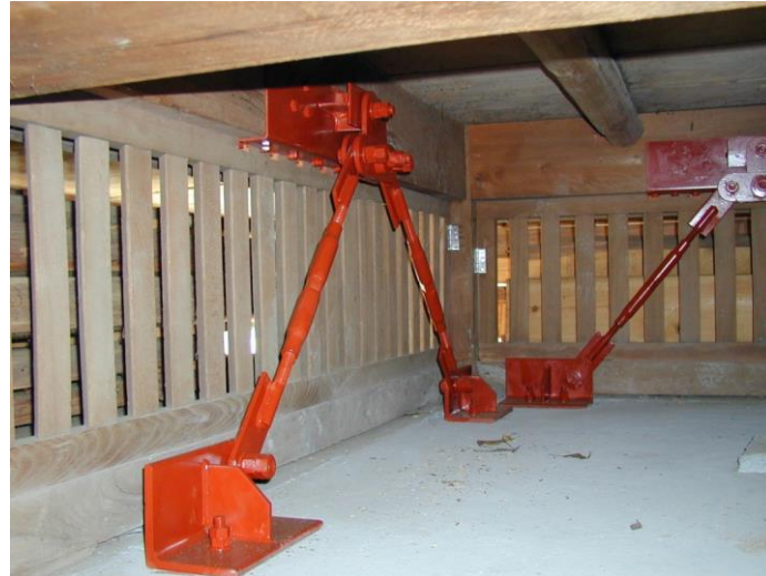
Figure 7 – Dampers with bracings installed in Yagutji Temple
