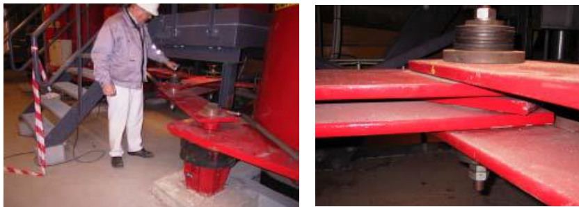
Figure 33- Friction damper devices for a simultaneous control of two centrifugal machines.
