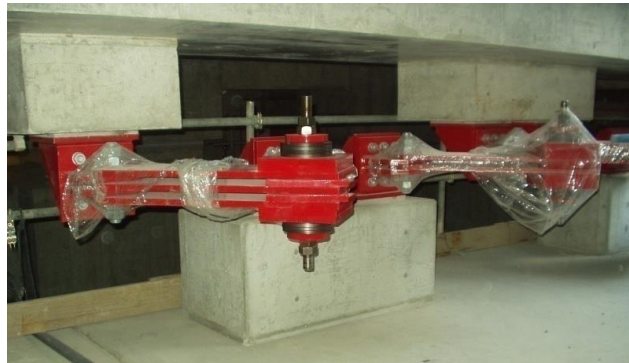
Figure 20 – Dampers installed in residential tower on Osaka
