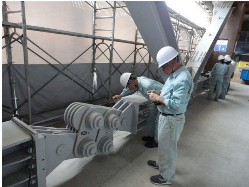
Figure 26 - 2250 kN Dampers installed in the tallest building in Japan
