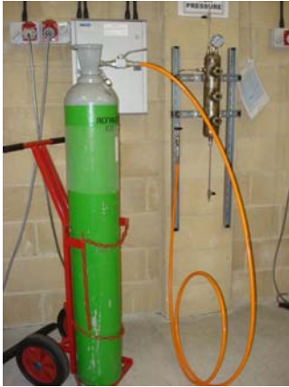
Figure 10, cylinder connected to charging equipment
