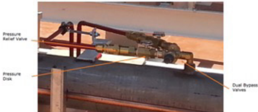
Figure 10. Close-up of additional protective devices.
