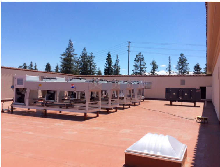
Figure 4. The seven propane units on the roof of the Santa Clara store
