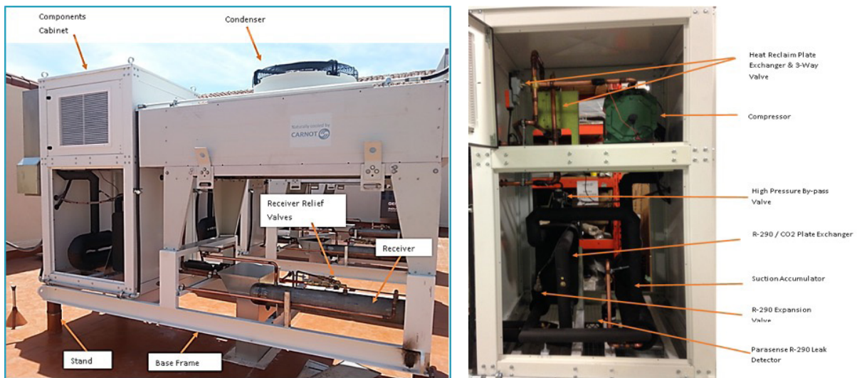
Figure 7. Rooftop refrigeration unit with detail.
