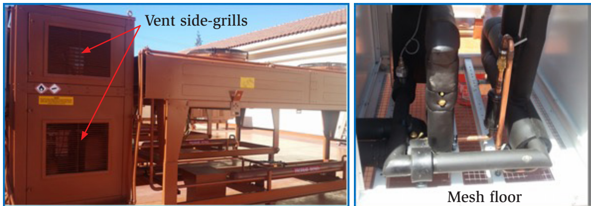
Figure 8. Passive safety features included in the Santa Clara installation.
