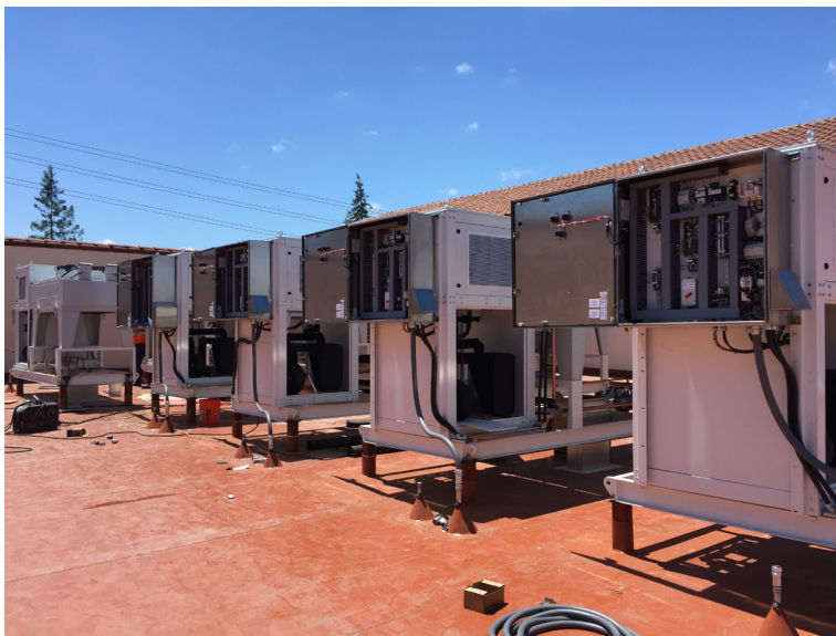
Figure 11. The electronic control panels on each propane unit.
