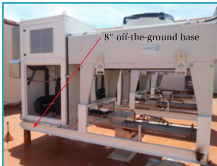
Figure 9. Refrigeration system support stands.
