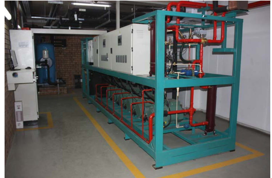
Inside the machine room of SPAR Wonderpark.
