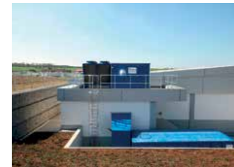
Fig. 2 Photo of Outdoor Integral Chiller Plant Installation
