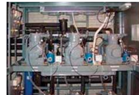
Fig. 2 Ahold Supermarket, Netherlands
