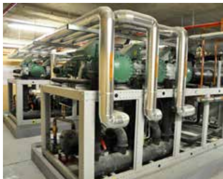
Fig. 3 System Installation of the Refrigeration System
