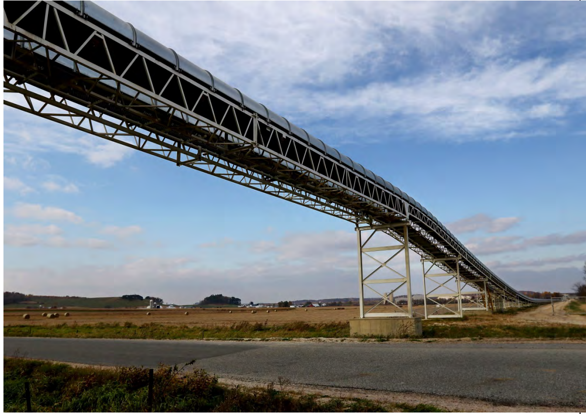
Figure 1-11 Industrial sand conveyor system in near Augusta, WI (photo: Dan Reiland, Leader Telegram website)
