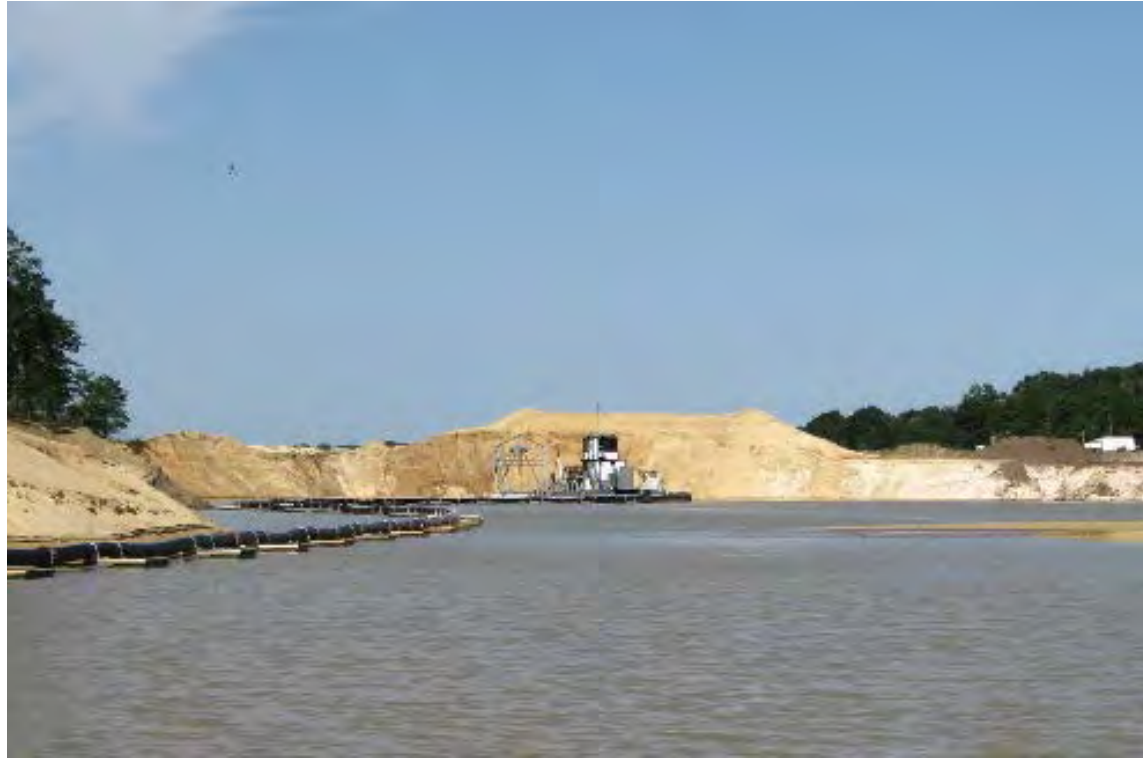
Figure 1-9 A hydraulic dredge and suction line at an industrial sand mine (photo Roberta Walls, DNR)
