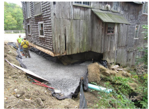
New sill and compacted crushed stone base under the south side of the ell. Photo by Bob Brown.
