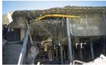
(k) Bullock's Department Store , 1994 Northridge Earthquake. Description of Structure: Waffle-slab floor-system supported on circular columns; opened in 1971. Damage Incurred: Punching shear failure of slab-column connections, followed by vertical collapse. Source: (Mitchell et al. 1995). Photo Credit: EERC Online Archive
