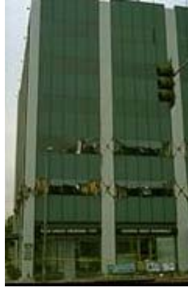
(j) Barrington Building , 1994 Northridge Earthquake. Description of Structure: 7-story non-ductile RC frame with discontinuous shear walls. Damage Incurred: Shear failure of most columns in 5 lower stories, due to spandrel beams that shortened columns, irregularity of shear walls and torsional effects. Columns did not lose their capacity to carry gravity loads. Source: (Mitchell et al. 1995; Youssef 1995) Photo Credit: EERC Online Archive
