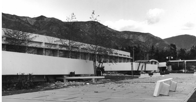
(c) Olive View Hospital Psychiatric Building, 1971 San Fernando Earthquake. Description of Structure: 2-story RC frame structure designed in 1965/1966; T-shaped configuration in plan. Damage Incurred: Entire 1 st story collapsed when columns failed in flexure-shear and then lost ability to carry gravity loads.
