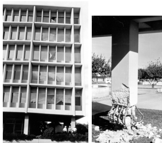
(f) Imperial County Services Building , 1979 Imperial Valley Earthquake . Description of Structure: 6-story RC frame building designed in 1968, with some discontinuous shear walls in upper stories. Structure
