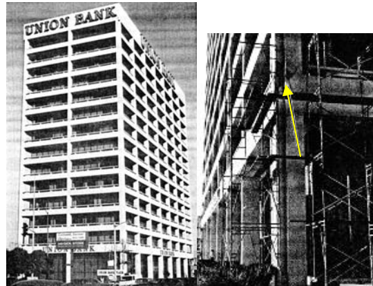
(e) Union Bank Building , 1971 San Fernando Earthquake . Description of Structure: 13-story RC frame structure. Damage Incurred: Cracks in columns in lower levels and damage to corner columns due to overturning effects. This structure was damaged again in the Northridge Earthquake. Source: (Frazier et al. 1971; Jennings 1971; Lew et al. 1971; Murphy 1973; Steinbrugge et al. 1975) Photo Credit: (Lew et al. 1971)
