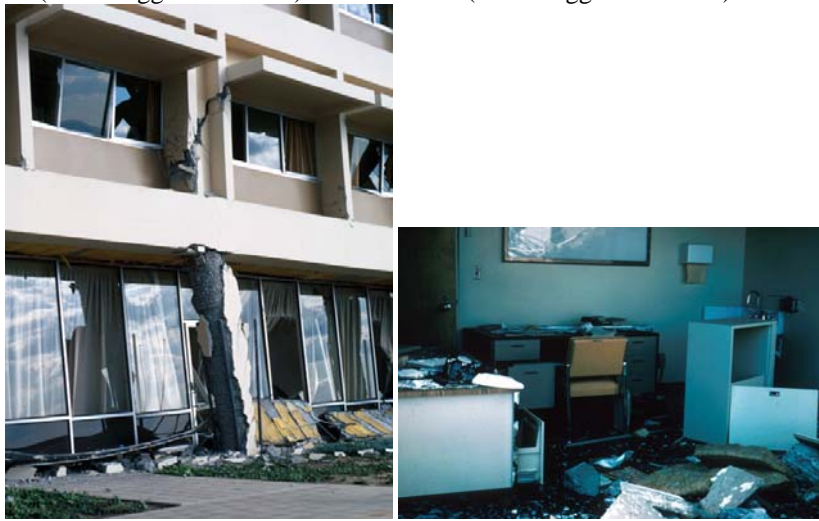
(b) Olive View Hospital Medical Treatment Building, 1971 San Fernando Earthquake. Description of Structure: 5-story building with lateral system consisting of RC Frames and shear walls, completed in 1970. Structure was very close to the epicenter of the earthquake and peak ground accelerations at the site probably exceeded 0.6g. Damage Incurred: Extensive damage in 1 st story and basement due to discontinuous walls and soft-story effect. Failure in columns occurred due to lack of confinement. Pounding occurred with neighboring buildings. Building was replaced following the earthquake (100% loss). Source: (Frazier et al. 1971; Jennings 1971; Lew et al. 1971; Murphy 1973; Steinbrugge et al. 1975) Photo Credit: USGS Photographic Library
