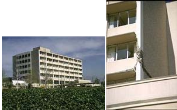
(d) Holy Cross Hospital , 1971 San Fernando Earthquake . Description of Structure: 7-story RC structure with RC frame lateral resisting system and shear walls in transverse direction, completed in 1961. Damage Incurred: Failure in beam-column joints and connection between framing, floor and wall systems. Source: (Frazier et al. 1971; Jennings 1971; Lew et al. 1971; Murphy 1973; Steinbrugge et al. 1975) Photo Credit: EERC Online Archive
