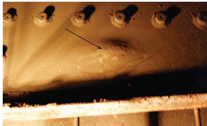
A bulging side sheet is an indication of overheating resulting from excessive scale buildup, as shown in this image of the inside firebox side sheet of 'Camila.'
