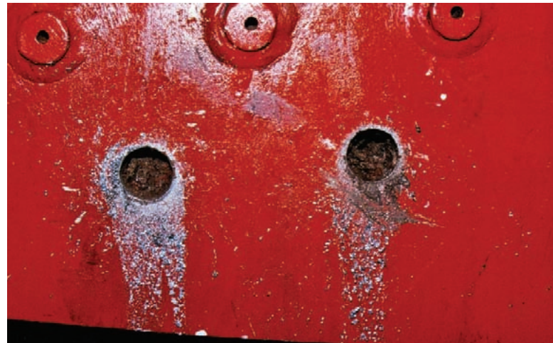
Holes drilled in the outer firebox reveal a water space nearly completely encrusted with scale and mud. This is the inverse side to the photograph of the bulge shown on PAGE 9.
