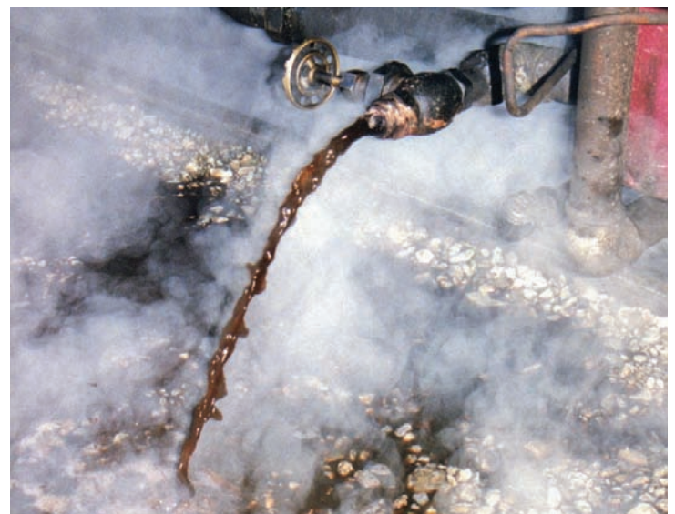
Even darker brown is acceptable , as is evident with this image of just-off-of-steam hot boiler water draining from the boiler of 'Camila.' With PT, the levels of TDS required are not harmful to the boiler.
