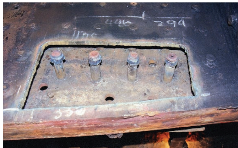
With a chunk of steel removed for making a patch , this image shows the corrosion on the sheets resultant from poor water treatment.
