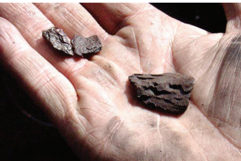
Following the initial application of PT, these large chunks of scale began to wash out of 'Camila's' boiler. The high pH level of the boiler water, combined with other chemicals, stripped this scale from the boiler.
