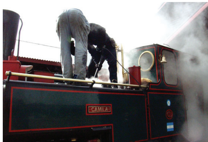
Step 2: Hot Power Wash the Boiler after the boiler water has been drained, a high-output steam cleaner is used to wash all interior surfaces of the boiler reachable from strategically-placed wash out plugs.
