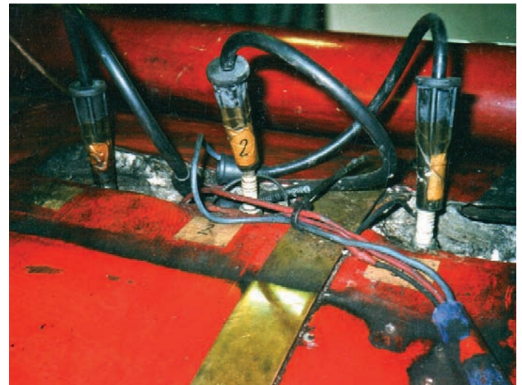
Once installed in the boiler , the electrodes feed a central processing unit that indicates whether water (or foam) is in contact with the end of the device. This informs crews as to whether the antifoam is adequate.
