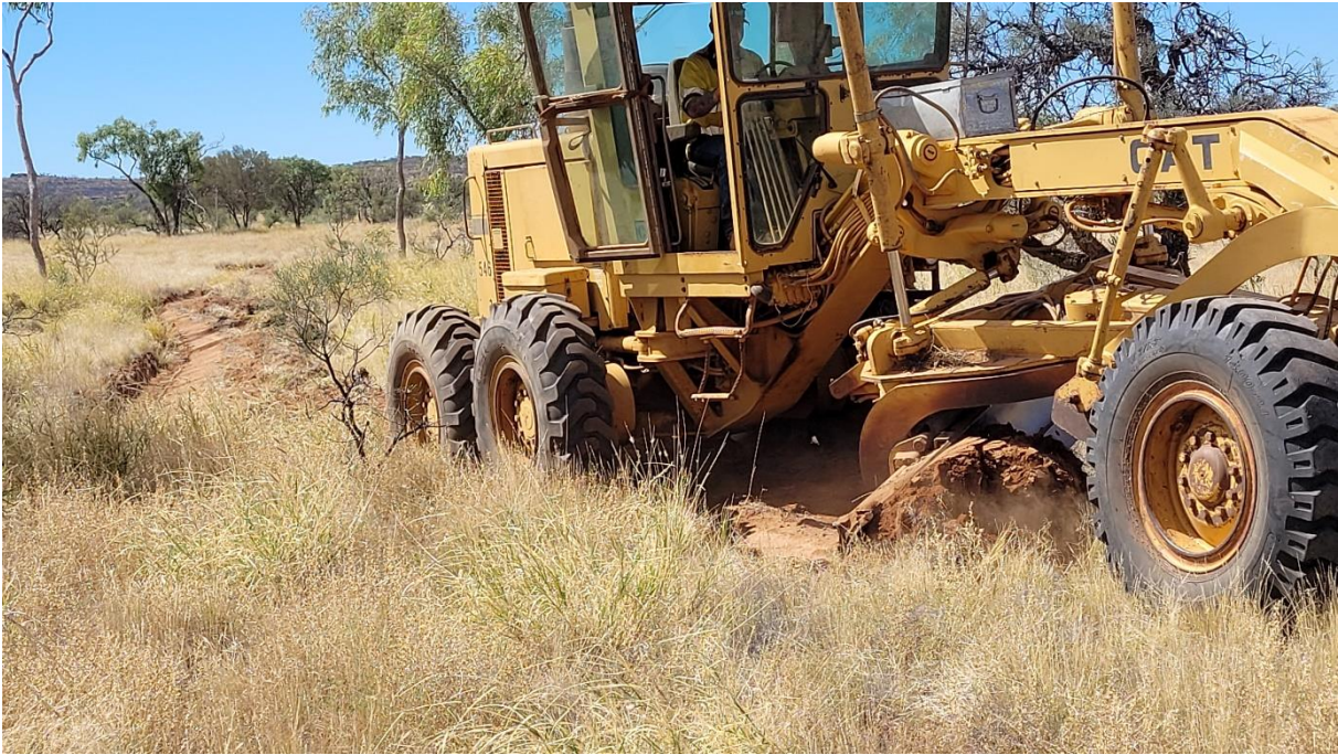
Figure 33 First pass of constructing a contour bank (note blade is pushing spoil downslope).
