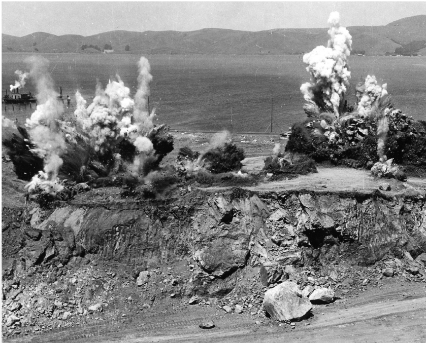
LEFT: This dramatic photograph shows Pine Point—now stripped of its buildings and trees—being blown up. The tons of dirt loosened by the explosions were quickly bulldozed to fill in the salt water marsh to the north that would soon become the hard, flat surface of the 202-acre Marinship boatyard.
