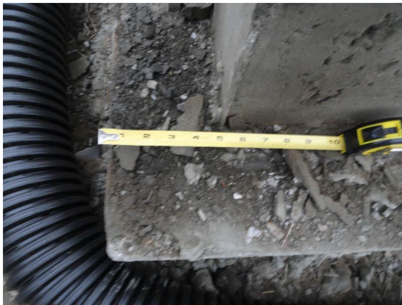
Figure 1 - The Project Manager will be required to place a ruler over the footings to demonstrate the width.
