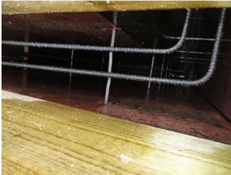
Figure 2 - A picture is to be taken inside the foundation to show the installation of rebar prior to concrete pour
