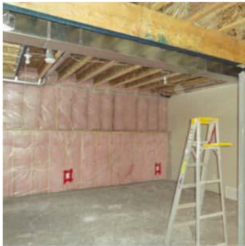
Figure 3 - A picture is to be taken to show the air barriers are sealed.
