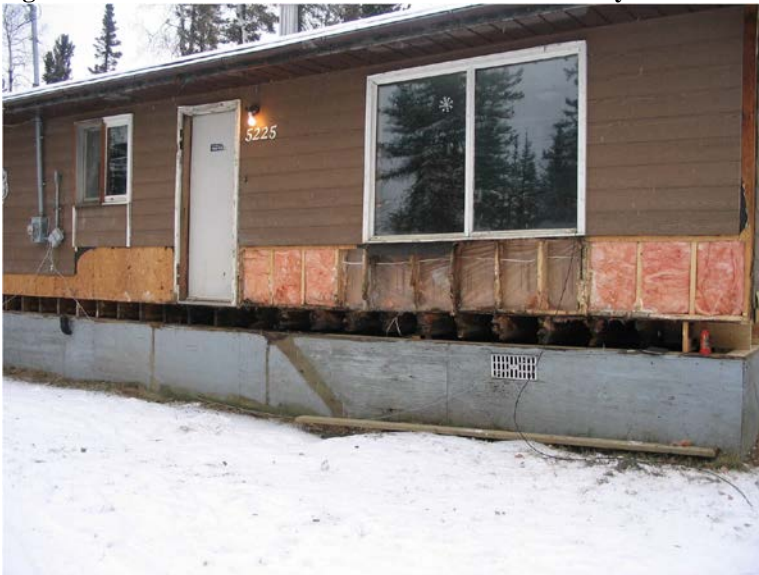
Figure 5 A home not properly constructed
