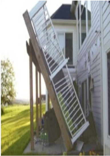
Figure 6 Collapsed railing from porch
