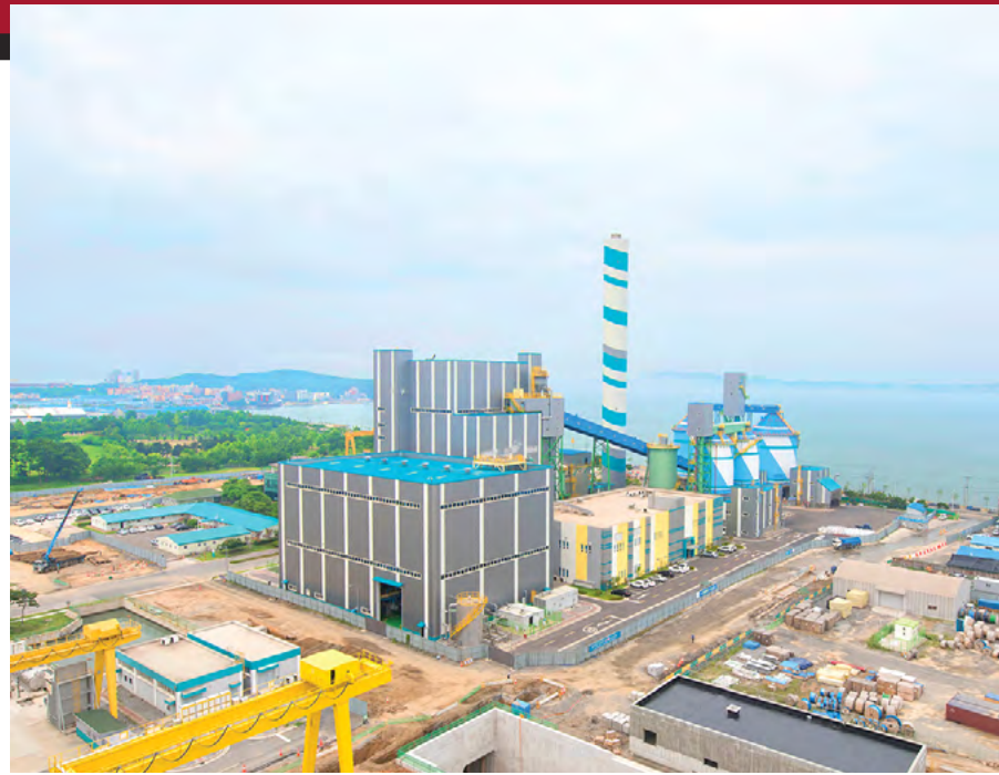
Dangjin Bio-1 in South Korea, which features our multi-fuel CFB technology, produces 105 MWe of power from palm kernel shells, wood pellets and recycled wood chips.
