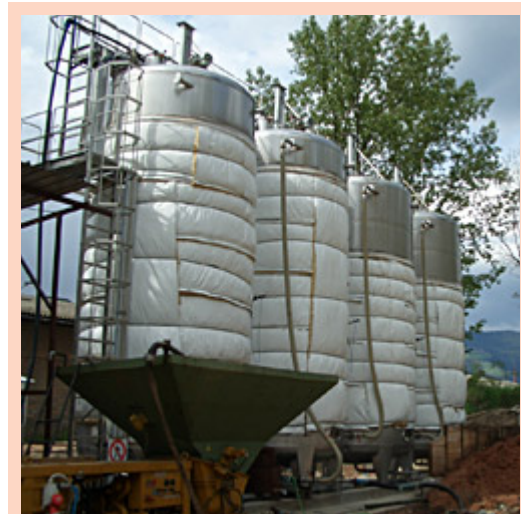
Biogas reactors at brickwork Gasser/Italy
