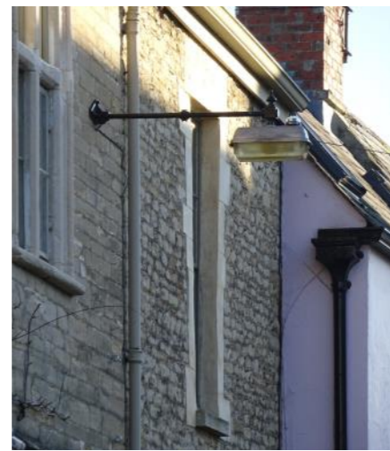
Figure 3.41: Mid 20th century wall mounted street lighting on Gloucester Street, is slim-lined and unobtrusive. This style of wall mounted fitting is still fairly common in the older parts of the town and should be retained where possible.
