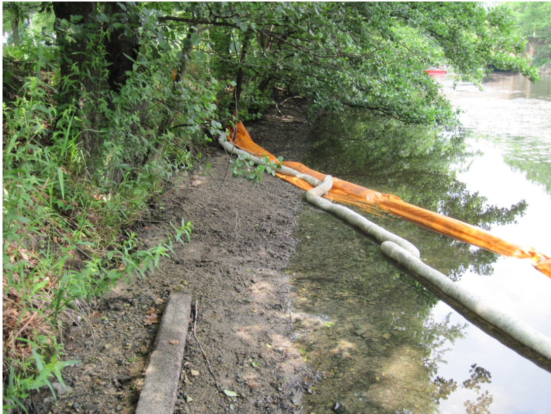
Photograph 24: View of station 0625-1725 (Area 675') during removal of impacted sediments/moss and water washing. Photograph taken on June 26, 2013.
