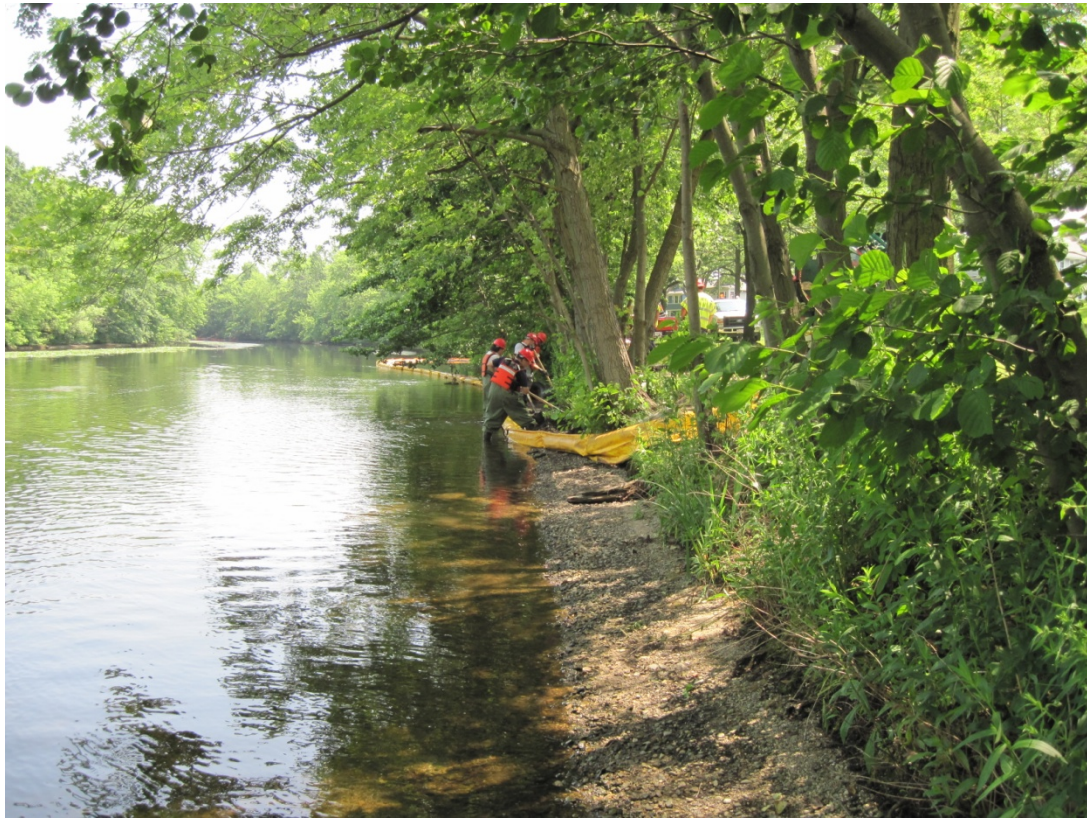
Photograph 21: View of station 1750-1850 (Area 1795') during removal of impacted sediments/moss and water washing. Photograph taken on June 25, 2013.
