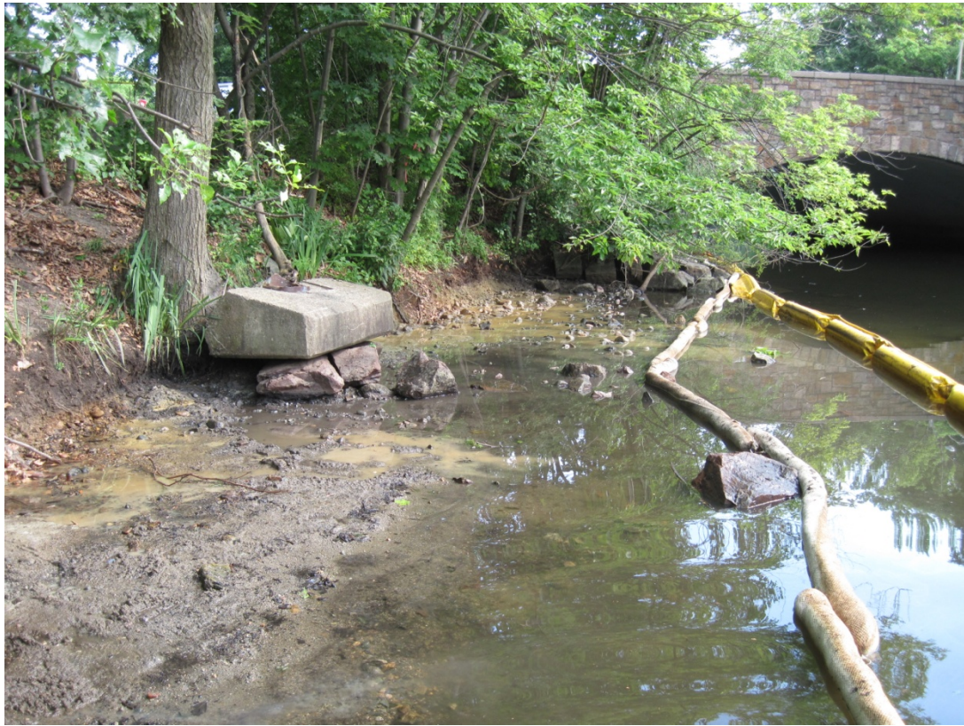
Photograph 25: View of station 0354 to 500 (Medford Street bridge) during removal of impacted sediments/moss and water washing. Photograph taken on June 26, 2013.
