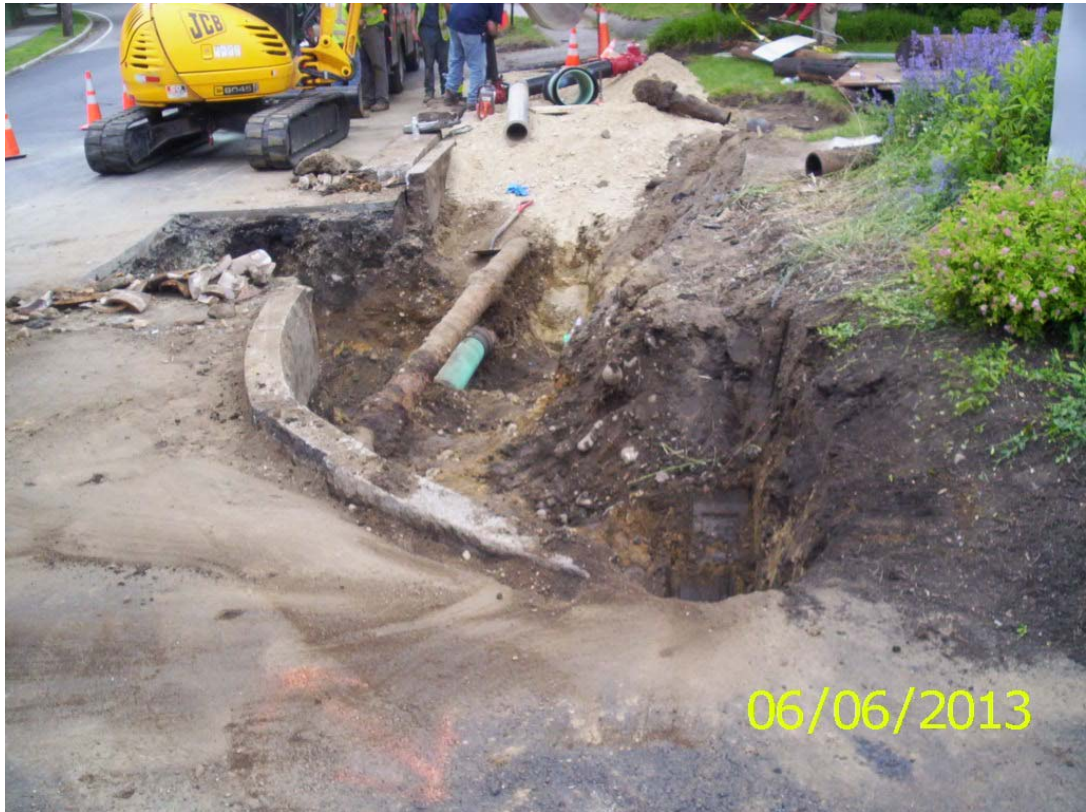
Photograph 17: View of completed excavation in front of Winchester Savings Bank. Photograph taken on June 6, 2013.
