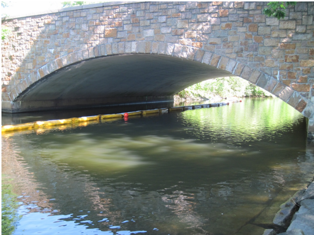
Photograph 14: View of absorbent and containment boom at Medford Street bridge during flushing of drain line. Photograph taken on June 5, 2013.
