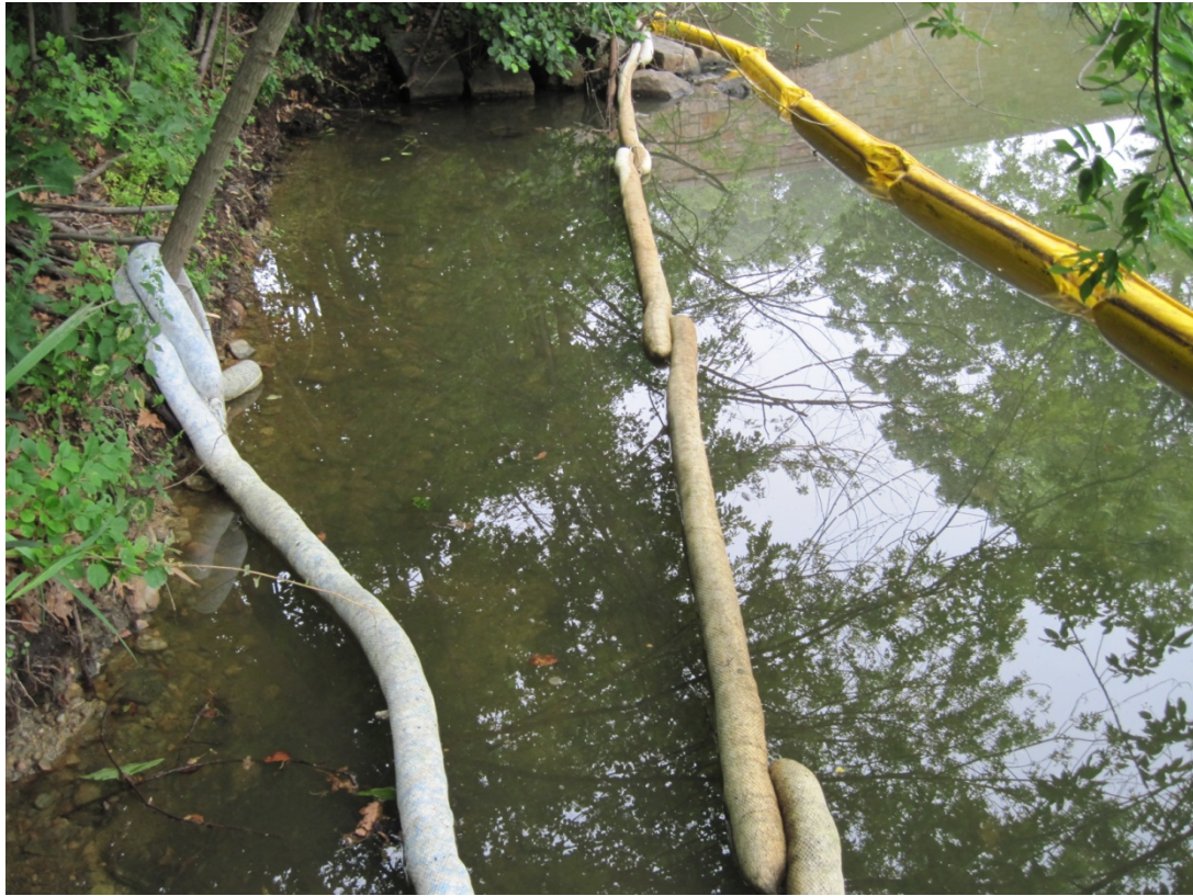
Photograph 27: View of absorbent and containment boom at Station 0354-0500 (Medford Street bridge). Photograph taken on July 10, 2013.
