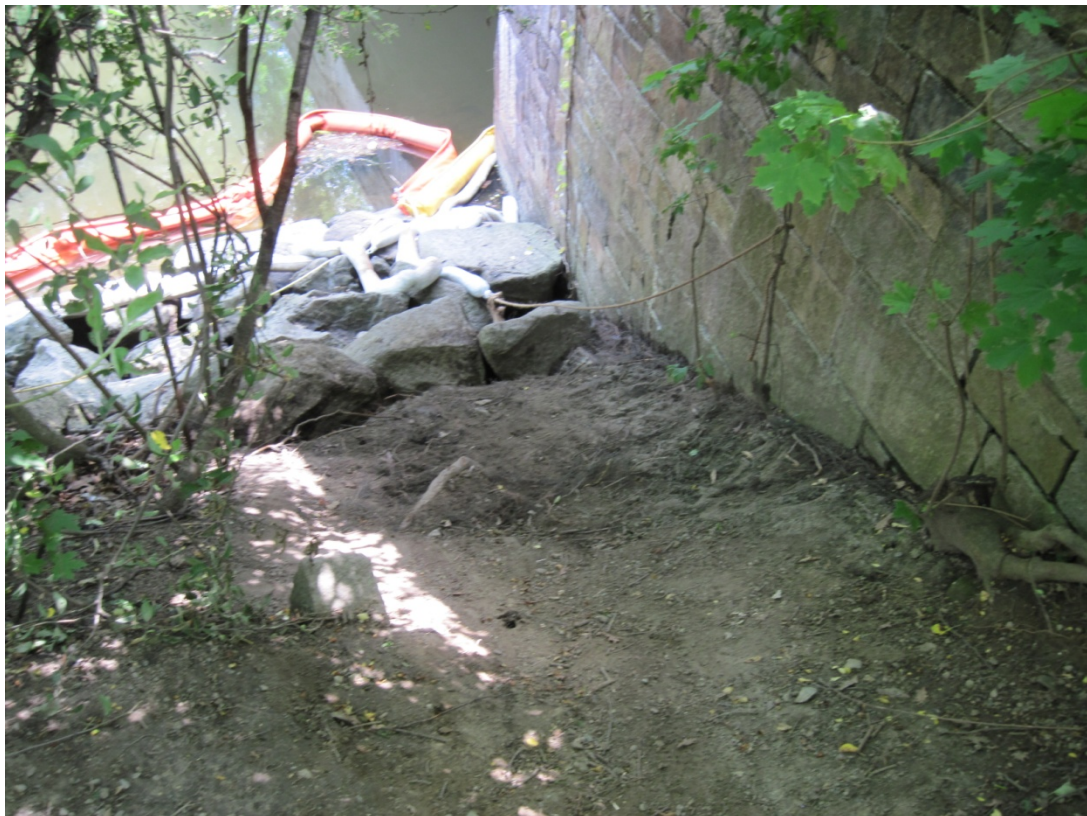
Photograph 26: View of completed excavation at rip rap above River Street bridge. Photograph taken on June 26, 2013.
