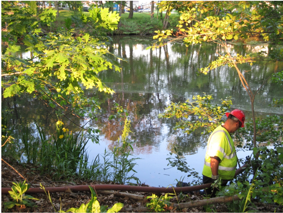
Photograph 3: View of product recovery activities in Mystic River downstream of the Medford Street bridge. Photograph taken on May 31, 2013.
