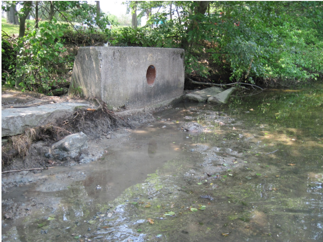
Photograph 22: View of station 1900-2000 (Boom 3 Collection Area, 1950') during removal of impacted sediments/moss and water washing. Photograph taken on June 25, 2013.
