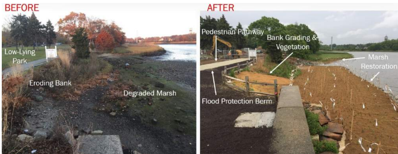
Figure 3. Watson Park Shoreline Erosion Mitigation and Coastal Resiliency Project – Before (left) and After (right), Spring 2022
