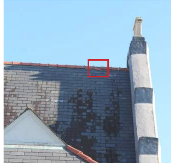
Figure 4.20: Damaged ridge cap. Photo by Cody Ellis, 2015.
