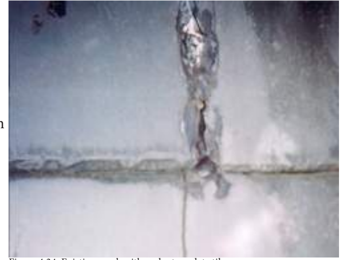
Figure 4.34: Existing crack with sealant on slate tile Photo courtesy of Dimitri Roby, 2014.
