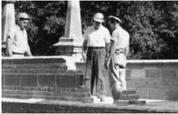
Construction underway on new cloister between chapel and parish house. c. 1959. Collection of Christ Church Cathedral.
