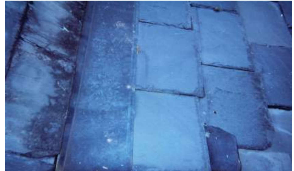
Figure 4.17: Broken shingles. Courtesy of Dimitri Roby, 2014.
