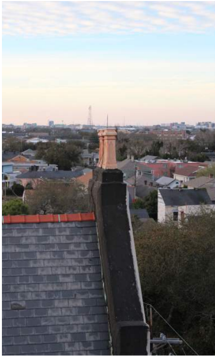
Figure 4.22: Tarred parapets. Photo by Cody Ellis, 2015.
