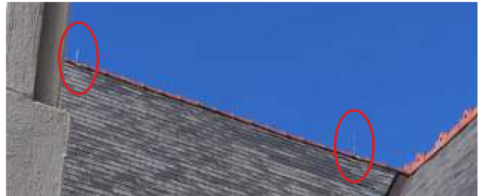
Figure 4.42: Existing lighting rods on the cathedral roof Photo courtesy of Cody Ellis, 2015
