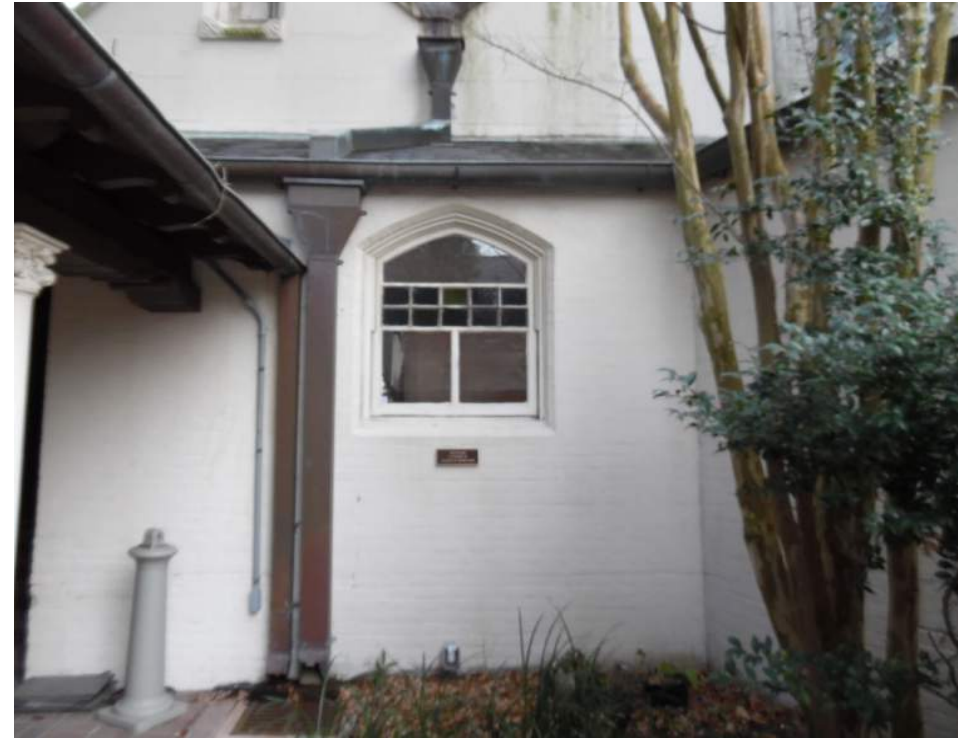
Figure # 6.8: Leader heads are positioned at and fitted to the tops of downspouts, allowing water to enter from different angles and minimizing overflow. This image from the Bishop's Garden shows leader heads attached to downspouts along two tiers of roof. Photo by Trudy Andrzejewski, 2015
