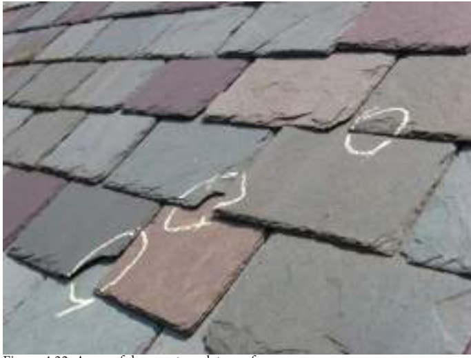
Figure 4.32: Areas of damage to a slate roof Source: http://0.tqn.com/w/experts/Roofing-1598/2010/10/Roof-Shot_1.jpg
