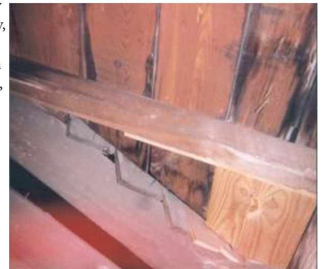
Figure 4.21: Nails protruding through sheathing. Courtesy of Dimitri Roby, 2014.
