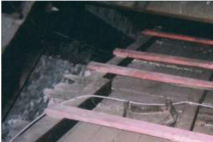
Figure 4.33: Current water damage in vault Photo courtesy of Dimitri Roby, 2014.
