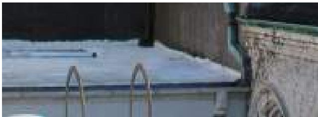
Figure 4.36: Built up tar edge around flat roof Photo courtesy of Cody Ellis, 2015
