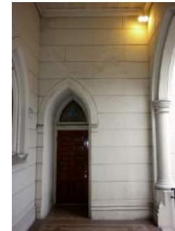
Figure 2.14: Picture of the Cathedral Portico Showing a Crack Above the Door. Photo by Matthew Cerick. 2015
