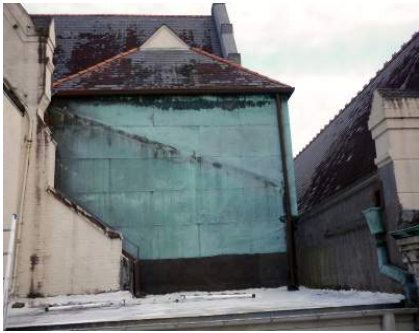
Figure 2.19 Picture of the Carondelet Street Elevation Cathedral Showing Water Damage on the Facade and Showing the Copper Plating. Photo by Matthew Cerick. 2015
