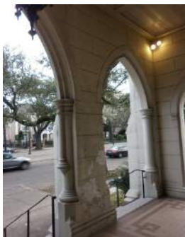
Figure 2.12: Picture of the Cathedral Portico Showing Blistering. Photo by Matthew Cerick. 2015
