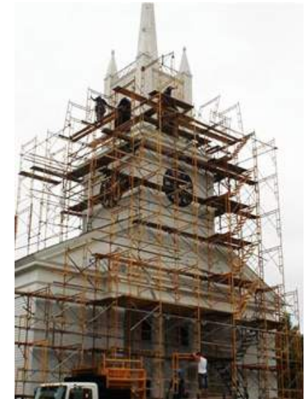
Figure 2.22 Photo depicting the scaffolding required to paint a church facade and bell tower. Photo credit to First Congregational Church of Rowley, MA.
