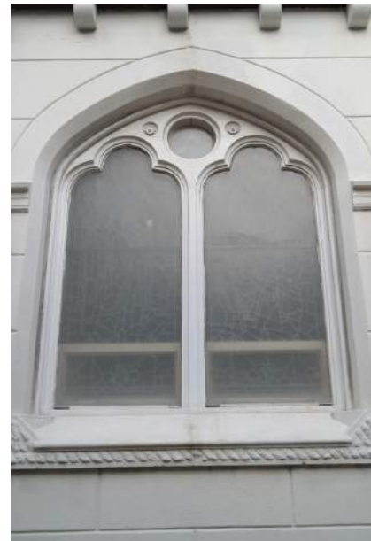
Figure 3.19: Non-vented opaque/failed protective glazing example on West Cathedral wall. All photos on this page credited to Samantha Williams
