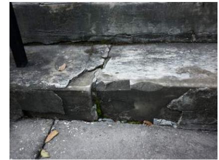
Figure 2.8: Picture of the St. Charles Avenue Elevation Chapel Steps Showing Cracks. Photo by Matthew Cerick. 2015
