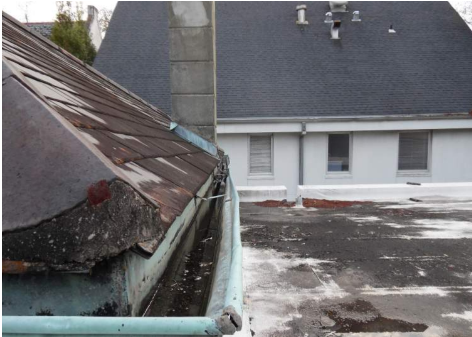
Figure # 6.6: Standing water in the copper gutters on a hipped roof behind the chapel and the adjacent flat roof. Photo by Trudy Andrzejewski, 2015
