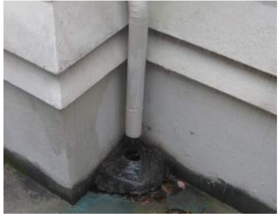
Figure # 6.10: This downspout is inadequately connected to the subterranean drain. Photo by Nathan Lott, 2015
