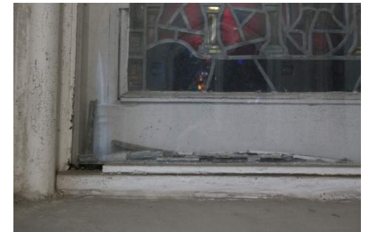
Figure 3.20: Sealant failure and debris visible behind glazing system. Window on East Chapel Wall, by Cathedral western entrance.
