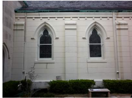
Figure 2.6: Picture of the Seventh Street Elevation of the Chapel Showing Cracks Under the Windows. Photo by Matthew Cerick. 2015
