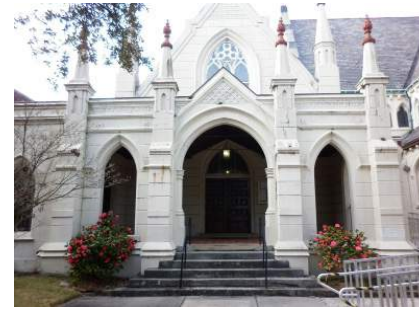
Figure 2.7: Picture of the St. Charles Avenue Elevation of the Chapel Showing Cracks. Photo by Matthew Cerick. 2015
