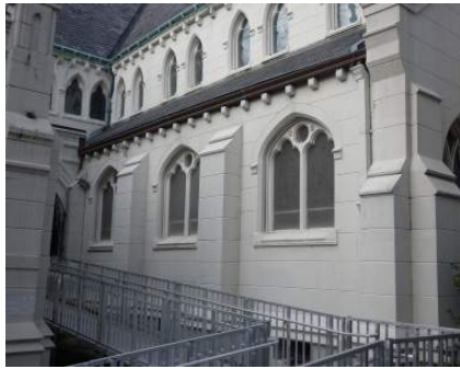
Figure 2.10 Picture of the Seventh Street Elevation Cathedral Showing Water Damage on the Recessed St. Charles Avenue Portion of the Facade Cornice. Photo by Matthew Cerick. 2015
