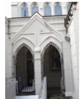
Figure 2.9: Picture of the St. Charles Avenue Elevation Between the Chapel and Cathedral Steps Showing Water Damage. Photo by Matthew Cerick. 2015
