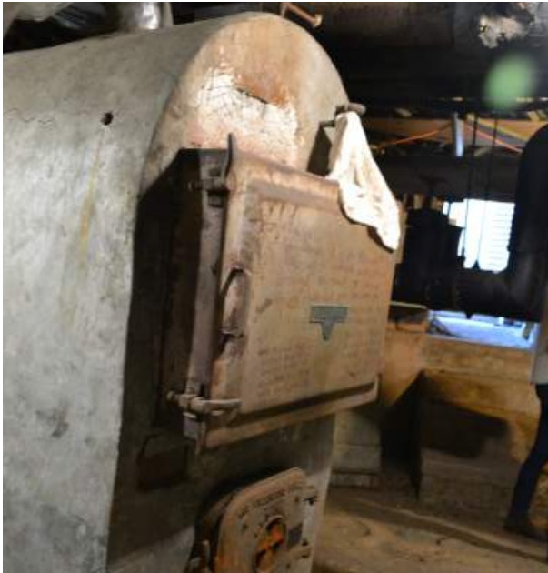
Figure 8.18: Fitzgibbons boiler of Christ Church Cathedral, part of the original active heating system. Photo by author.
