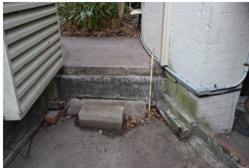
Figure 7.20: Grade change from Mechanical Yard to Bishop's Garden of 18 inches, photo by Amanda Keith, 2015
