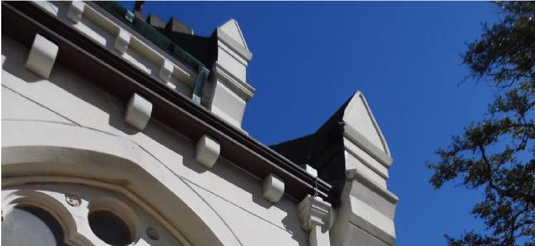
Figure # 6.1: A section of K gutter on the lower level of the Nave roof. Photo by Trudy Andrzejewski, 2015
