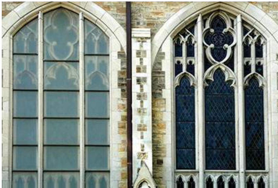
Figure 3.15: Left window shows protective glazing without regard for tracery and the right window was restored and the protective glazing removed. Credit: Neal A. Vogel and Rolf Achilles via The Preservation and Repair of Historic Stained and Leaded Glass
