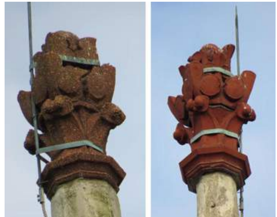
Figure 5.5-5.6 : Tower Finials: in poor condition on the left and fair condition on the right. Photos by Laura Stokley, 2015
