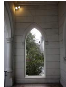
Figure 2.13: Picture of the Cathedral Portico Showing a Crack Above the Window. Photo by Matthew Cerick. 2015
