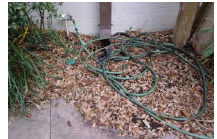
Figure 7.18: Drain clogged with plant matter in bed against ambulatory, Bishop's Garden, photo by Amanda Keith, 2015
