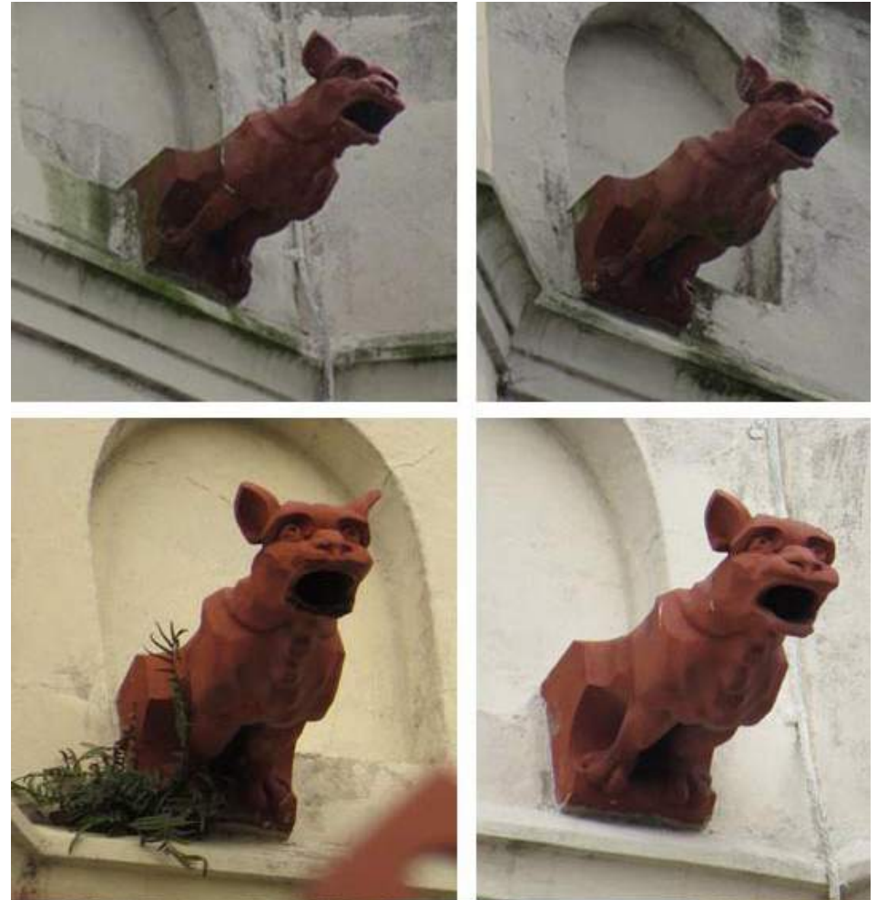
Figure 5.17-5.20 : Tower gargoyles showing bio growth, ferns and staining. Photo by Laura Stokley, 2015
