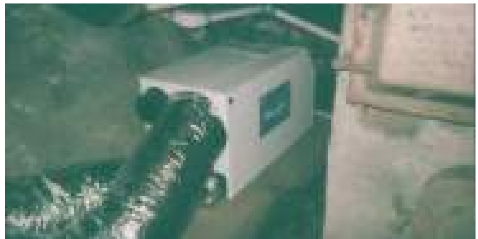
Figure 8.17: Current active cooling system. Photo by Dimitri Roby.
