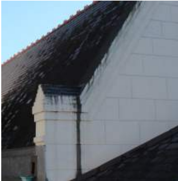
Figure 4.39: Tar covered parapits over chapel Photo courtesy of Cody Ellis, 2015
