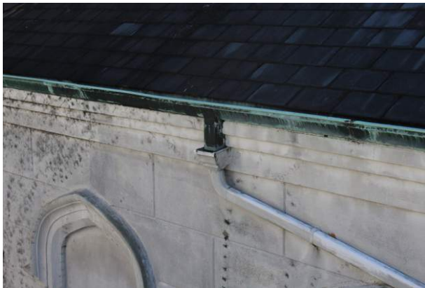
Figure 4.19: Damaged gutters. Photo by Cody Ellis, 2015.
