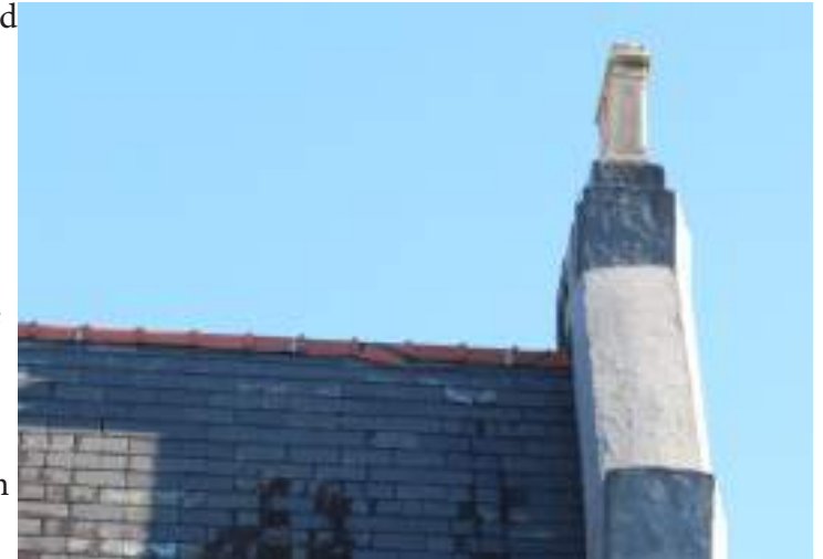
Figure 4.37: Broken finial on north ridge Photo courtesy of Cody Ellis, 2015
