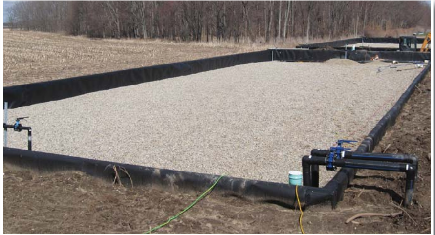
Mentone's SAGR (Submerged Attached Growth Reactor).
