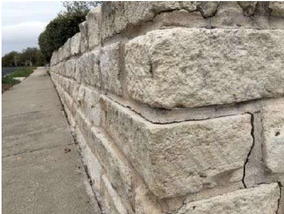
Each row of this retaining wall is slightly set back from the layer below it.
