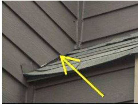
Photo 10-6 Flashing visible from rear yard.
