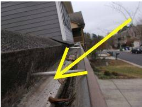
Photo 11-1 Front gutters are improperly sloped such that water is being retained inside the gutters. The standing water is 'wicking' into the soffit causing moisture intrusion.
