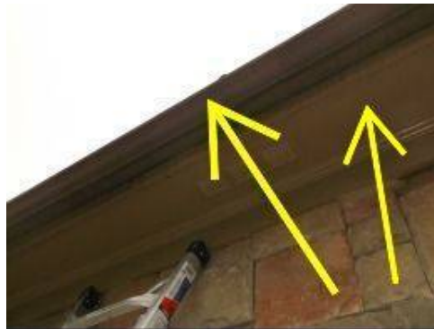
Photo 5-16 Soffit shows signs of moisture intrusion due to water standing inside the gutters.
