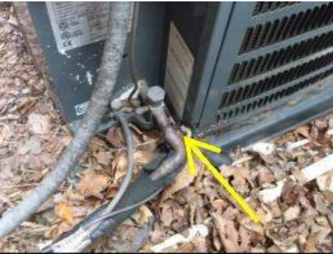
Photo 24-1 Air Conditioning refrigerant lines have insulation deteriorated. Replace as necessary.
