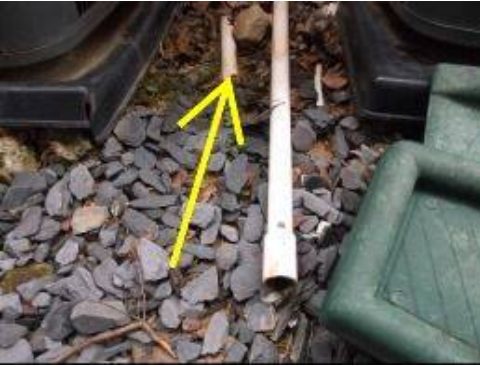
Photo 23-1 Clogged Air Cond. condensate line.
