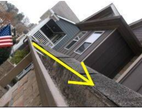
Photo 10-3 Water is standing inside the front gutters. The front gutters are improperly sloped.
