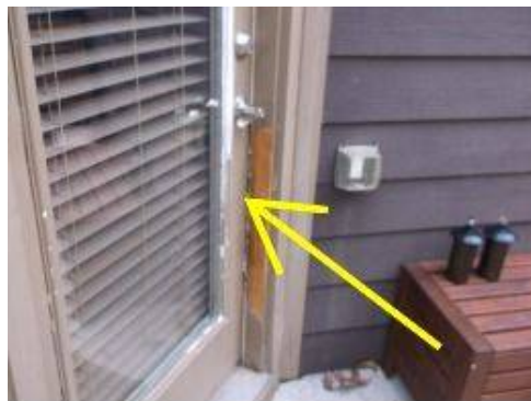
Photo 5-12 Rear patio door is damaged by pets. Repair as necessary.
