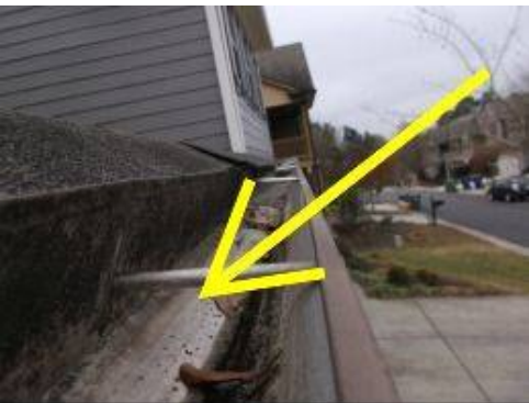
Photo 11-1 Front gutters are improperly sloped such that water is being retained inside the gutters. The standing water is 'wicking' into the soffit causing moisture intrusion.
