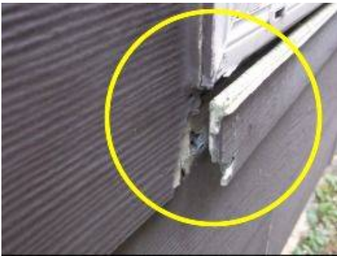
Photo 5-9 Exterior window trim is pulling away from the siding. Repair and re-attach with proper fasteners, caulk and seal joints.
