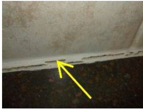
Photo 28-6 Kitchen counter-top has cracks in the caulking where the counter-top intersects with the back-splash.
