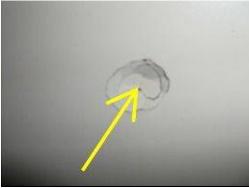
Photo 30-1 Impact damage to bedroom door in master bedroom.
