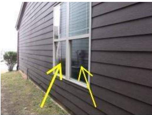
Photo 31-1 Exterior screens missing from several windows.
