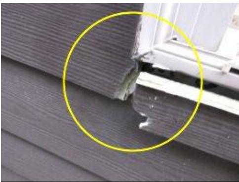
Photo 5-11 Repair and seal all siding butt joints and re-attach loose siding members.
