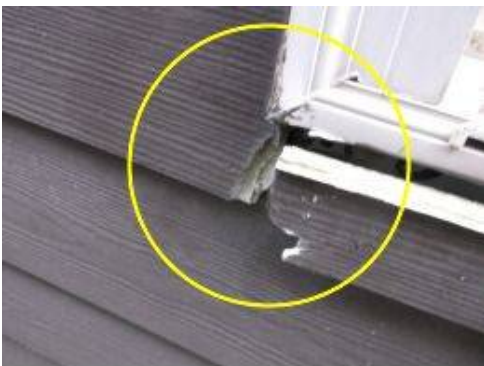
Photo 5-11 Repair and seal all siding butt joints and re-attach loose siding members.
