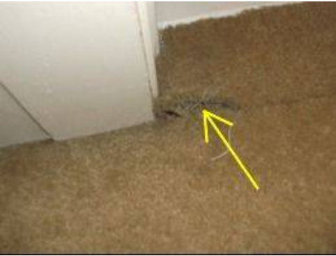
Photo 29-9 Carpet is torn at the seams at entrance to master bathroom. Repair as necessary.
