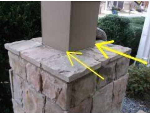
Photo 6-1 Mortar joints cracked at front porch support columns.
