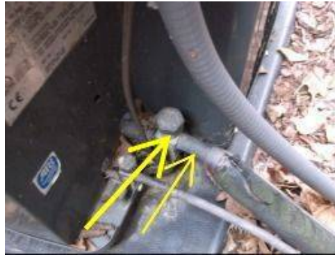
Photo 24-2 Insulation deteriorated at A/C unit refrigerant line.
