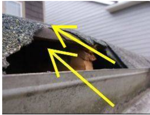
Photo 10-4 Roofing shingle at front entrance above garage has broken off and needs replacement. Contact qualified roofing company.
