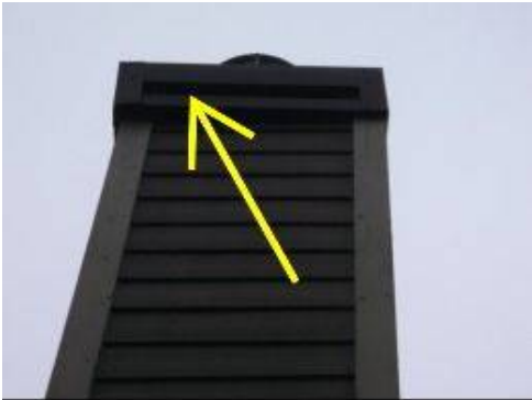
Photo 10-5 Metal chimney cap appears to be improperly installed from ground level. Further evaluation is recommended.
