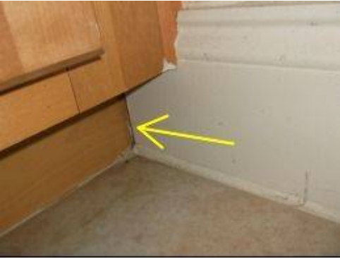
Photo 29-7 Caulk and seal joints at the bottom cabinet trim in the master bathroom.
