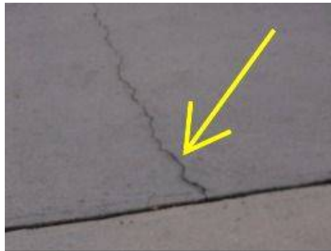
Photo 3-4 Minor crack in driveway.
