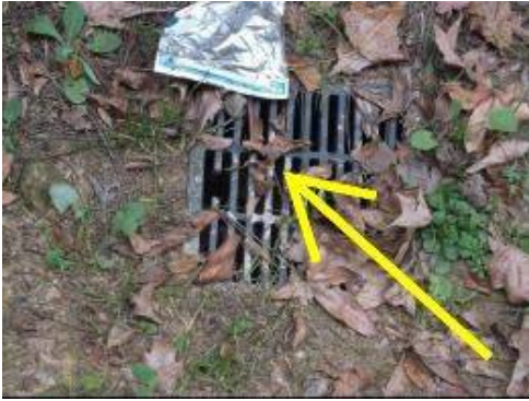
Photo 3-1 Yard drain is clogged with leaves and debris. Clean out drain to allow for proper drainage away from the foundation.
