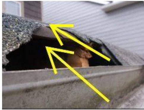
Photo 10-4 Roofing shingle at front entrance above garage has broken off and needs replacement. Contact qualified roofing company.
