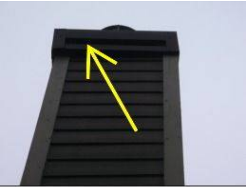
Photo 10-5 Metal chimney cap appears to be improperly installed from ground level. Further evaluation is recommended.
