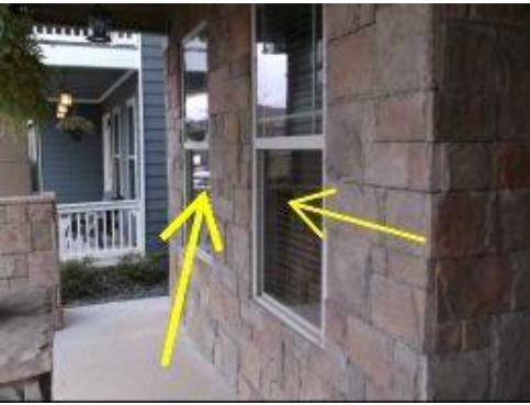
Photo 31-3 Exterior screens missing.
