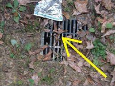
Photo 3-1 Yard drain is clogged with leaves and debris. Clean out drain to allow for proper drainage away from the foundation.
