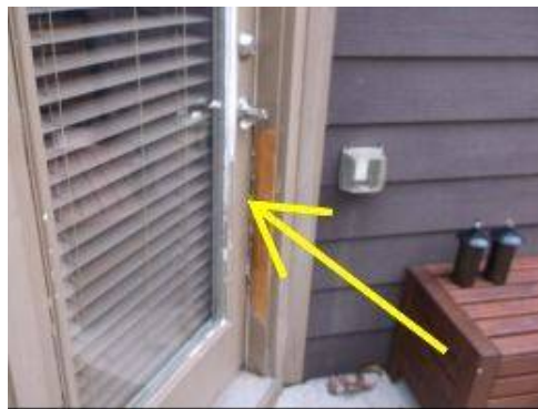
Photo 5-12 Rear patio door is damaged by pets. Repair as necessary.
