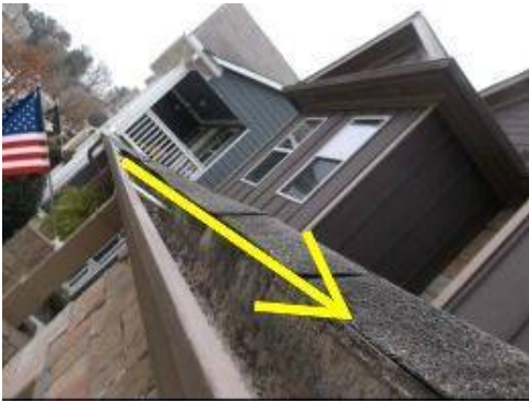
Photo 10-3 Water is standing inside the front gutters. The front gutters are improperly sloped.
