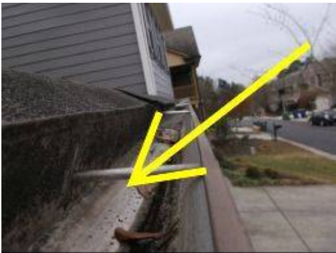
Photo 11-1 Front gutters are improperly sloped such that water is being retained inside the gutters. The standing water is 'wicking' into the soffit causing moisture intrusion.
