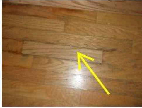
Photo 30-2 Laminate flooring in family room appears to have been repaired or a section replaced. Inquire of current owner or tenant if this is the case.
