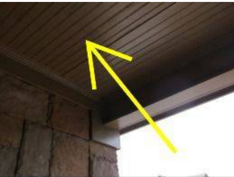
Photo 5-15 Front entrance porch ceiling appears to have mold spores forming. Recommend pressure washing with an anti-mold agent. This should be done periodically.....as the upper porch ceiling may not get adequate sunlight or ventilation to prevent moisture droplets from forming on the ceiling.
