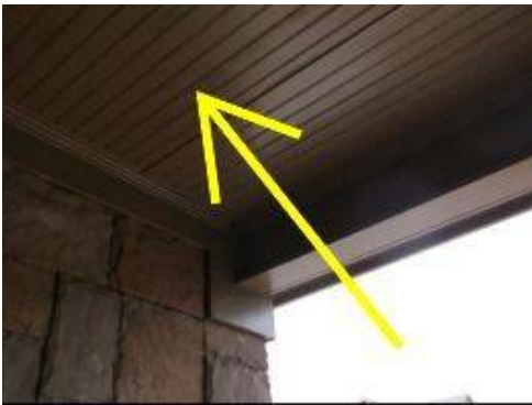
Photo 5-15 Front entrance porch ceiling appears to have mold spores forming. Recommend pressure washing with an anti-mold agent. This should be done periodically.....as the upper porch ceiling may not get adequate sunlight or ventilation to prevent moisture droplets from forming on the ceiling.
