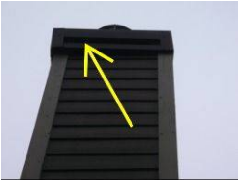
Photo 10-5 Metal chimney cap appears to be improperly installed from ground level. Further evaluation is recommended.
