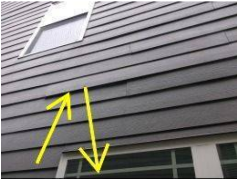
Photo 5-7 Siding member has pulled away from the substrate. It needs re-attached and repaired with the proper fasteners and sealed.
