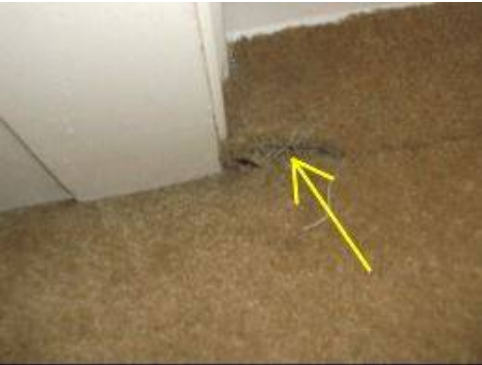
Photo 29-9 Carpet is torn at the seams at entrance to master bathroom. Repair as necessary.
