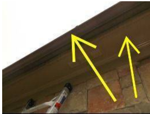
Photo 5-16 Soffit shows signs of moisture intrusion due to water standing inside the gutters.
