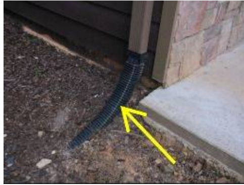
Photo 3-2 Downspout extension embedded in the soil. No discharge pipe was located during the inspection.
