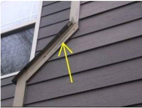
Photo 5-13 Siding trim is moisture damaged and dry-rot. Replace trim wood and re-paint with premium quality paint.
