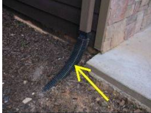
Photo 3-2 Downspout extension embedded in the soil. No discharge pipe was located during the inspection.
