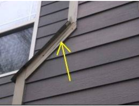
Photo 5-13 Siding trim is moisture damaged and dry-rot. Replace trim wood and re-paint with premium quality paint.
