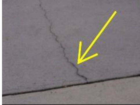
Photo 3-4 Minor crack in driveway.
