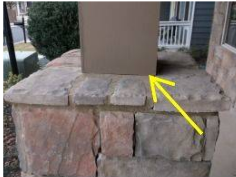
Photo 6-2 Minor cracks in the mortar joints at the front support columns.
