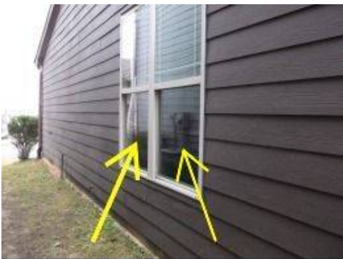
Photo 31-1 Exterior screens missing from several windows.
