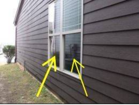
Photo 31-1 Exterior screens missing from several windows.
