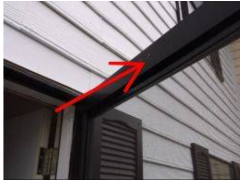
Photo X-8 Pneumatic door closer is missing from the storm door.
