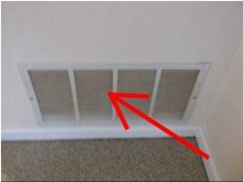
Photo X-7 The furnace air handler grill is dust and grease laden and needs a thorough cleaning.
