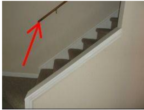
Photo X-6 No returns installed on the upstairs handrails. Open ends of stair handrails could cause sleeves to be caught on the ends and cause potential falls.
