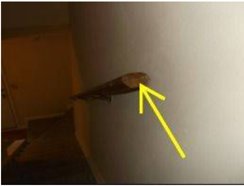
Photo X-5 The ends of stairwell handrails should have 'returns' at either end to prevent sleeves from getting caught on the ends and causing falls.
