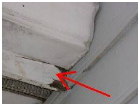
Photo X-10 Gutter is improperly sloped, and water standing inside the gutter is 'wicking' into the wood trim and fascia, causing moisture damage.
