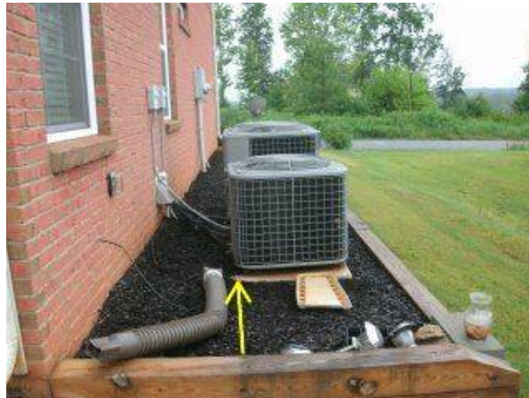
Photo 10-2 DOWNSPOUT EXTENSION AND SPLASH BLOCK NEED TO BE INSTALLED PROPERLY...TO PREVENT WATER FROM 'POOLING' UP AGAINST FOUNDATION.
