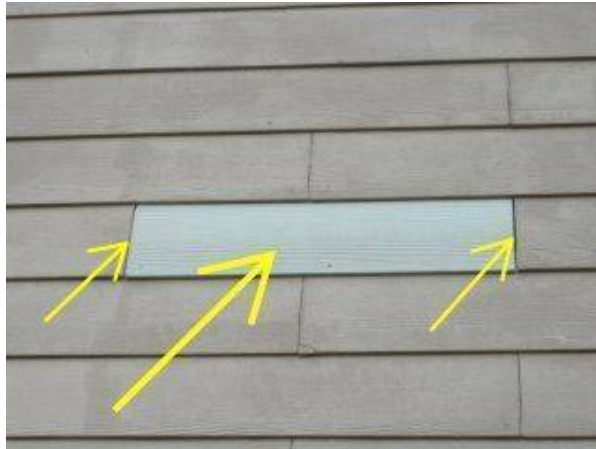
Photo X-14 THERE ARE SEVERAL EXTERIOR SIDING MEMBERS WHICH HAVE BEEN REPLACED AND RE-PAINTED AT SEVERAL LOCATIONS.
