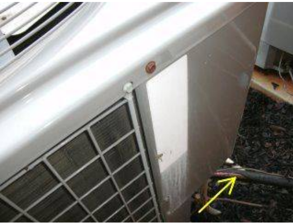
Photo X-15 AIR CONDITIONING REFRIGERANT LINE INSULATION IS PULLING AWAY FROM PIPES.
