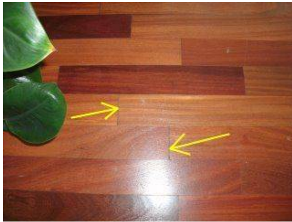
Photo X-16 GAPS OBSERVED IN HARDWOOD JOINTS IN FAMILY ROOM.
