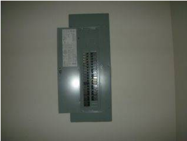
Photo X-13 GARAGE DOOR OPENER IS BEING FED BY A GFCI (GROUND FAULT CIRCUIT INTERRUPTER) TYPE RECEPTACLE. THESE OUTLETS ARE PRONE TO 'PHANTOM TRIPPING' AUTOMATIC DOOR OPENER MAY NOT ACTIVATE OCCASIONALLY...PARTICULARLY DURING INCLEMENT WEATHER.
