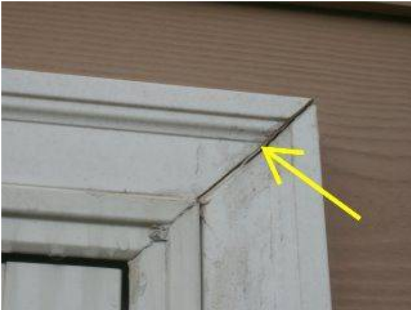
Photo X-5 WINDOW EXTERIOR TRIM ARE PULLING AWAY FROM MITRE JOINTS. CAULK AND SEAL WITH WEATHER-RESISTANT TYPE.
