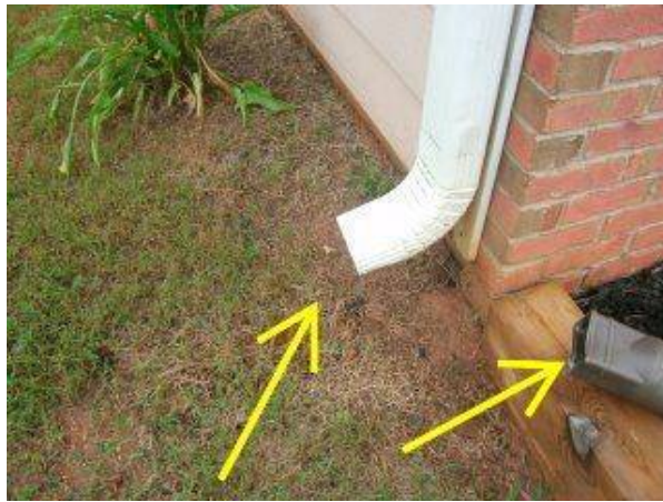
Photo X-22 DOWNSPOUT EXTENSIONS NEED TO BE RE-INSTALLED FOR PROPER DRAINAGE AWAY FROM FOUNDATION.
