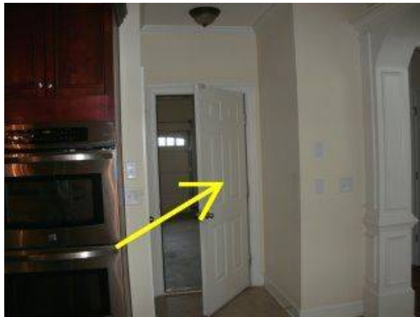
Photo X-20 THE DOOR THAT SEPARATES THE LIVING SPACE FROM THE GARAGE IS REQUIRED TO BE 'FIRE- RATED'. THIS DOOR DOES NOT APPEAR TO BE OF FIRE RATED MATERIAL.
