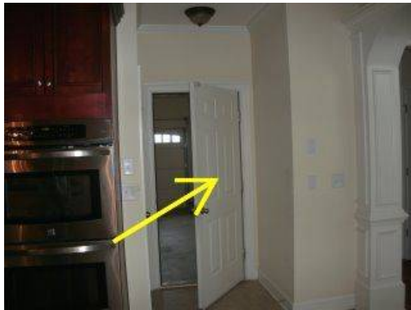
Photo X-20 THE DOOR THAT SEPARATES THE LIVING SPACE FROM THE GARAGE IS REQUIRED TO BE 'FIRE-RATED'. THIS DOOR DOES NOT APPEAR TO BE OF FIRE RATED MATERIAL.
