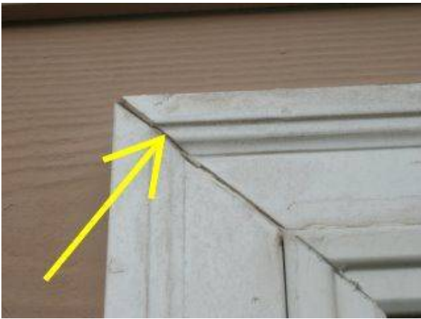
Photo X-21 GAPS BETWEEN TRIM JOINTS EXPOSE WOOD MEMBERS TO WEATHER. CAULK AND SEAL ALL EXTERIOR SIDING AND TRIM JOINTS.
