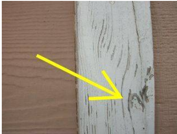
Photo X-18 SIDING TRIM PAINT IS PEELING AND EXPOSING WOOD TO WEATHER.
