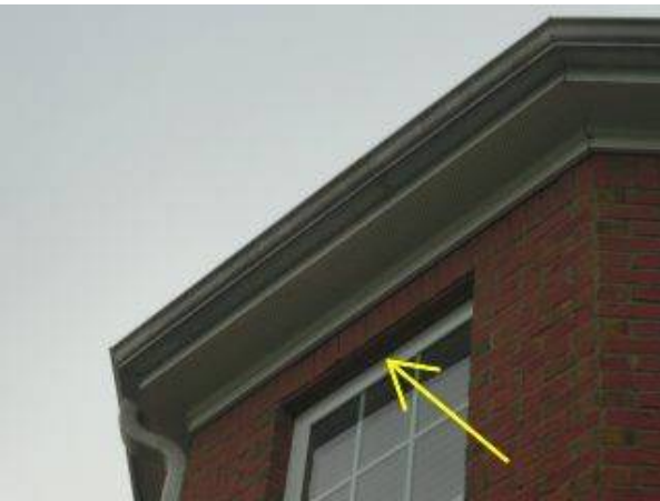
Photo X-19 CAULK AND SEAL ALL EXTERIOR SIDING JOINTS AND WINDOW TRIM TO PREVENT MOISTURE INTRUSION.
