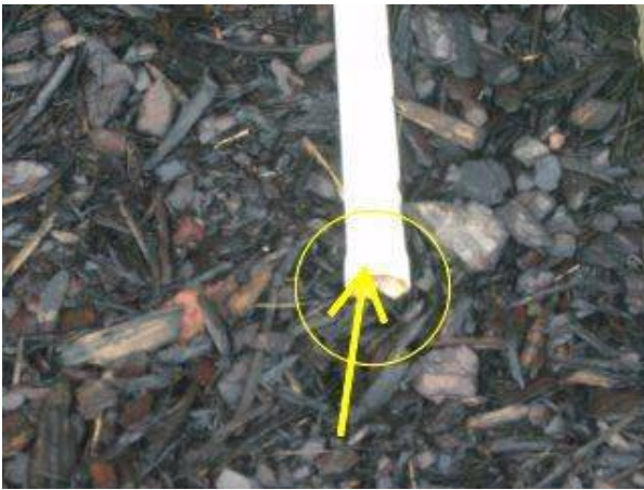
Photo 11-1 CLOGGED CONDENSATE LINES CAN RESULT IN MOISTURE RETENTION IN THE ATTIC.
