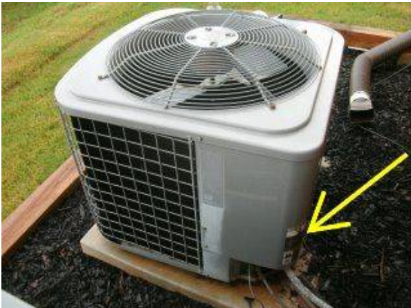
Photo 10-1 AIR CONDITIONER CONDENSER/COMPRESSOR UNITS SHOULD BE RAISED A MINIMUM OF 3" INCHES ABOVE GROUND AND RESTING LEVEL FOR OPTIMUM OPERATION.
