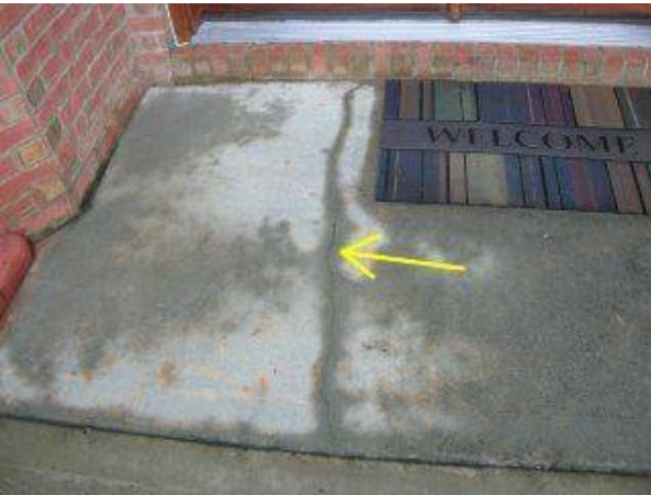
Photo X-17 MINOR CRACKS IN CONCRETE WALKWAY. THESE ARE COMMON AND DO NOT APPEAR TO BE SERIOUS.
