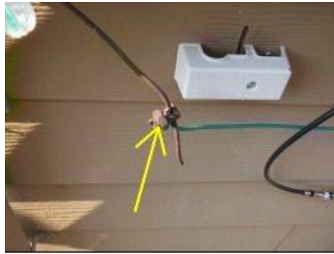
Photo X-6 The electrical ground wire is 'spliced' near the exterior panel box. Ground wires for the electrical system may not be spliced at any point along the wire.
