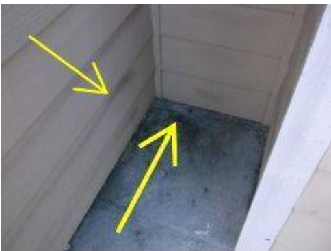
Photo X-9 There is evidence that water is being retained inside the corner of the rear concrete patio. There is suspected mold and algae growth on the siding at this location.
