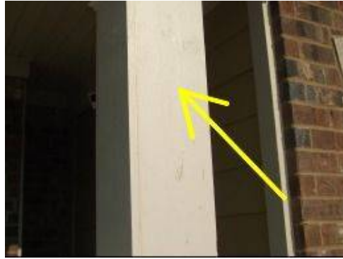
Photo X-12 Front porch support columns have peeling paint and minor splits in the wood members. Recommend re-painting with prime plus 2 coats of premium quality paint.
