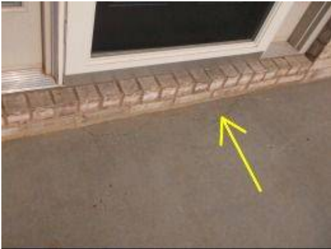
Photo X-3 Hairline cracks on the concrete porch at the entrance.
