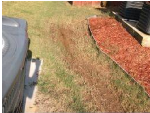
Photo X-30 Water is 'ponding' at the side yard nearest the air conditioning compressor units.
