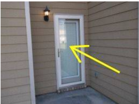
Photo X-43 Glass storm door could potentially be a hazard of persons colliding with the door when lighting is poor.
