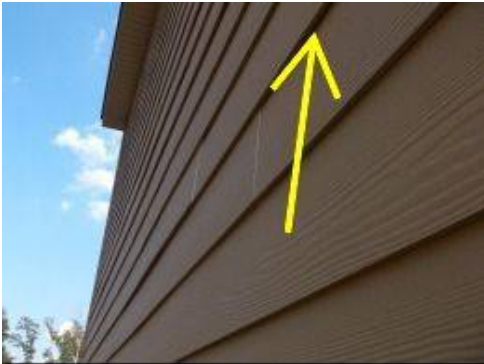
Photo X-7 Several siding members are 'loose' and need fasteners replaced.
