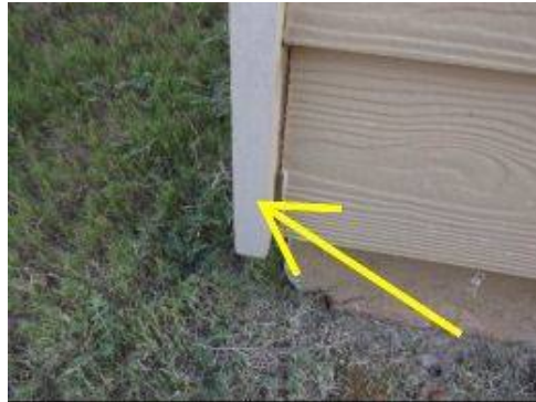
Photo X-8 Caulk and seal all siding and trim joints to prevent moisture intrusion. This corner trim piece is located at the back yard adjacent to the concrete patio. The trim is also split at several locations.
