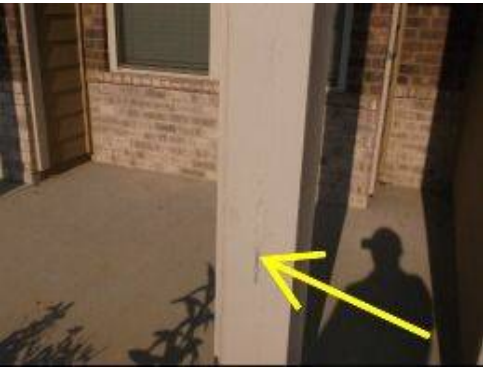
Photo X-11 Front porch support columns need re-painting with prime plus 2 coats of premium quality paint. Wood members are exposed to the weather. Re-paint where necessary.
