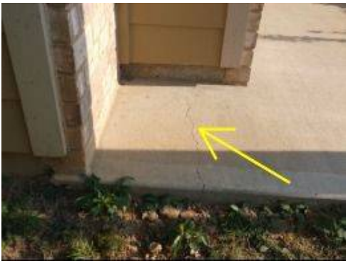
Photo X-19 Hairline cracks in the concrete porch at the front entrance.
