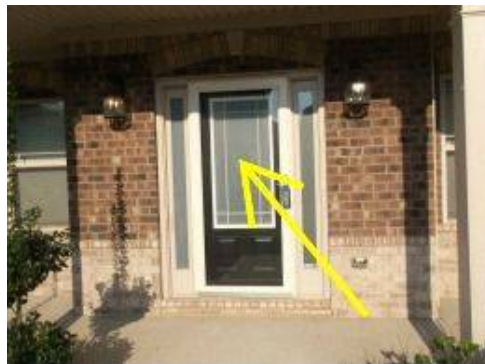
Photo X-44 Front entrance with glass storm door. The glass storm door could be a potential hazard of persons colliding with the door when lighting is poor.
