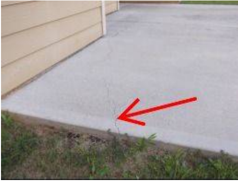
Photo 4-5 Hairline cracks observed at rear concrete patio surface.
