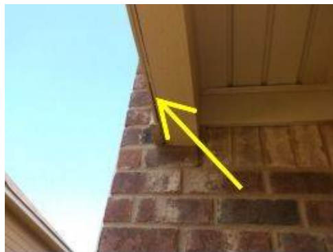
Photo X-10 Trim above front entrance concrete porch is pulling away from the siding.
