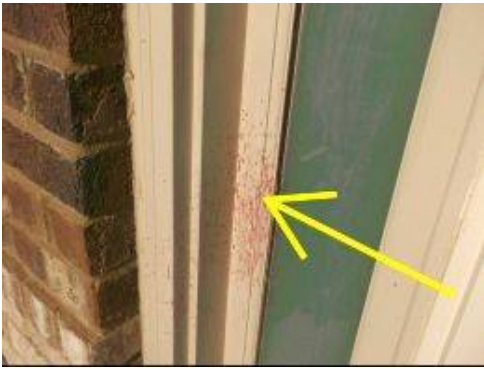
Photo X-39 There is a 'red' paint stain at the front entrance door trim.
