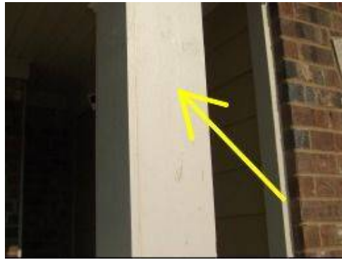
Photo X-12 Front porch support columns have peeling paint and minor splits in the wood members. Recommend re-painting with prime plus 2 coats of premium quality paint.
