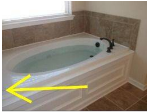
Photo 18-6 Master bathroom jetted tub does not respond to normal operating controls. The spring loaded on/off switch is defective.
