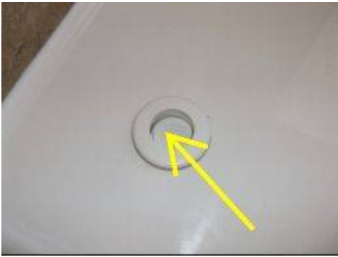
Photo 18-5 Jetted tub switch motor does not engage. The spring loaded switch is defective. Repair and/or replace and test as necessary.
