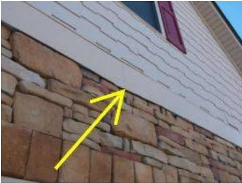
Photo 9-1 Drip flashing above garage door is not properly installed. Aesthetically uneven.
