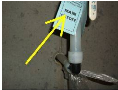
Photo 18-8 Main water shut-off located in basement. This valve shuts off water to plumbing fixtures in the entire house, should it become necessary to interrupt service in an emergency.
