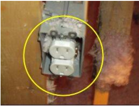
Photo 16-1 Cover plate missing from attic duplex receptacle exposing live energized parts.
