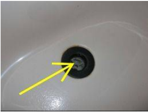
Photo 26-3 Bathroom stopper is missing from upstairs bathroom.
