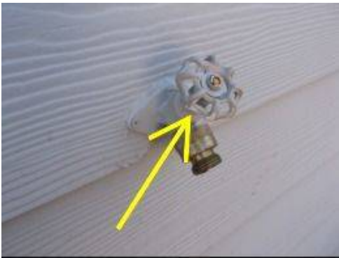
Photo 18-7 Exterior hose bib is split and leaking when valve is opened.
