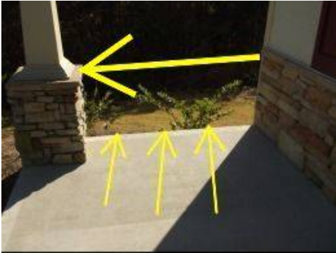
Photo 13-1 All unenclosed surfaces 30 inches or higher requires guardrails to prevent occupants from falling off and potential injury. Recommend guardrails be installed at the side entrance porch.
