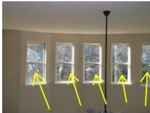
Photo 28-2 Windows above family room need cleaning. Paint or mortar stains visible from floor level.
