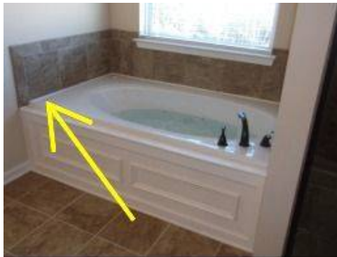
Photo 18-2 Jetted tub motor does not respond to normal operating. The switch is defective and the motor does not engage. Repair and test as necessary.
