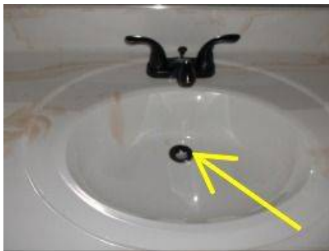
Photo 18-4 Upstairs bathroom sink stopper is missing. Replace as necessary.
