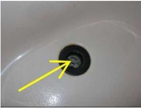
Photo 26-3 Bathroom stopper is missing from upstairs bathroom.
