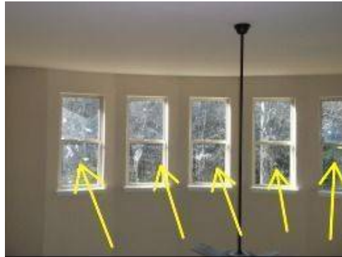
Photo 28-2 Windows above family room need cleaning. Paint or mortar stains visible from floor level.
