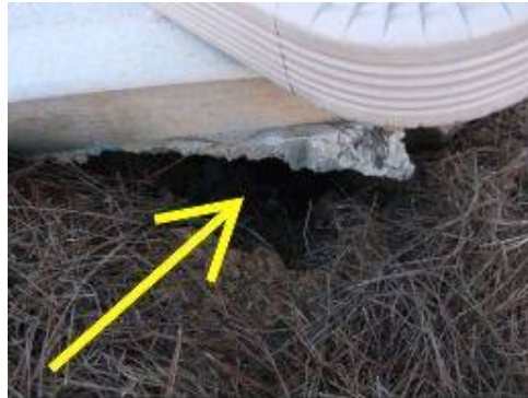
Photo 9-2 A portion of the concrete driveway base and footing is not fully supported by the ground. There is a large hole where the concrete meets the ground surface. The unsupported concrete could potentially collapse and break off affecting the remaining concrete surfaces. This area appears to not be properly and fully back-filled.
