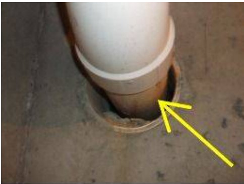
Photo 18-1 Recommend caulking and sealing of all wall penetrations from the basement walls.
