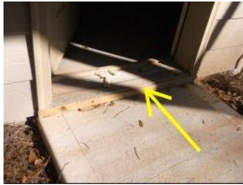
Photo 10-2 Wood kick plate in contact with concrete landing. Untreated lumber should not be in direct contact with concrete surfaces, due to the potential for rot.
