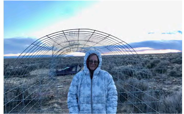
First Day of Desert Fish House Build Welded Steel Livestock Panels, April 2021
