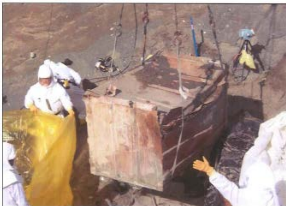
Hanford waste being removed from a burial ground, to be sent to Perma-Fix Northwest. Photo from WA Department of Ecology report. 22
