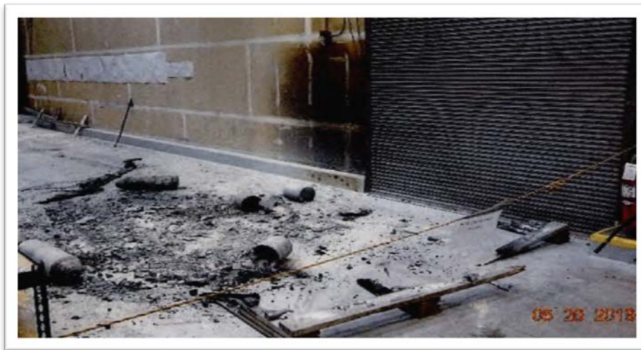
Remnants of fire in GeoMelt Room (Source: Washington Ecology Department, see footnote 57))
