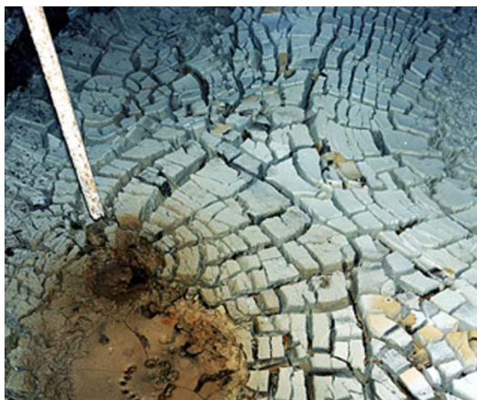
Figure 1 Hanford Tank U-104. One Example of grout/cement failure. i
