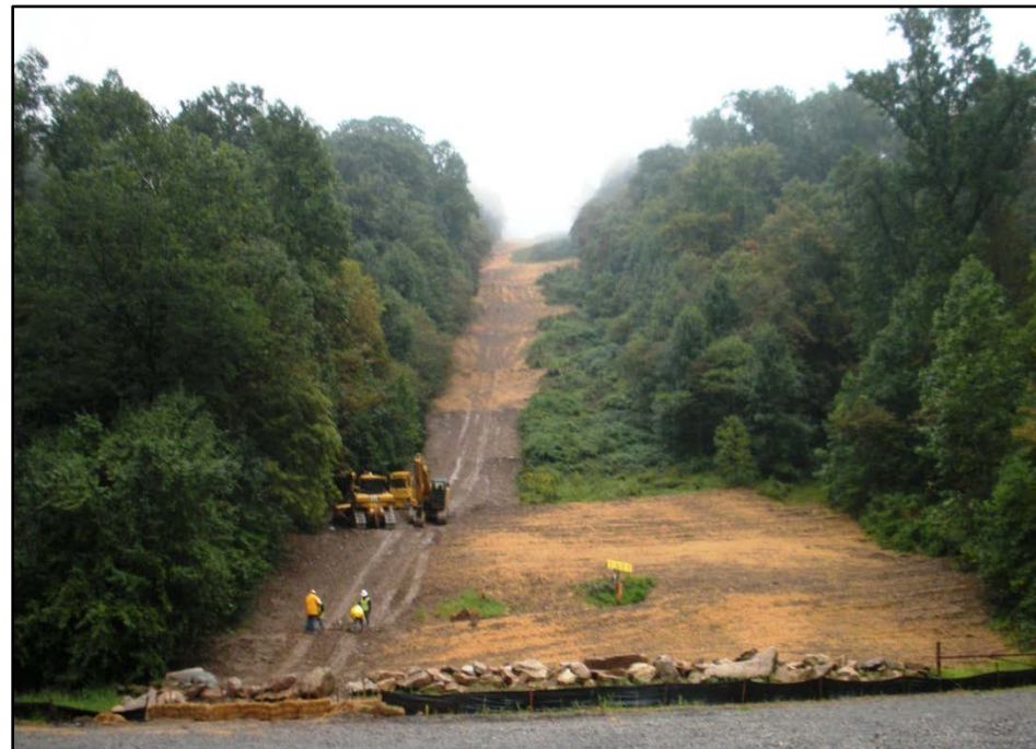
Photo 6: Natural Gas Transmission Pipeline, Dunbar Township, PA, Fayette County.
