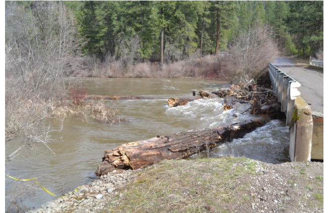
BIA Bridge is now repaired from damage caused by a log jam behind bridge at Twenty One Mile Road, located in northern Sanpoil Valley.
