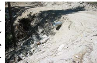
Unstable road fill eroding into stream. (Sleepy Hollow)
