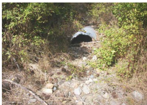
Partially plugged culvert
