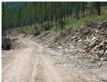
Groundwater interception by road causing erosion
