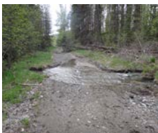
Road washout at Beaver Dam Creek.
