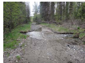
Road washout at Beaver Dam Creek
