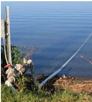
Oxygenation System at Twin Lakes
