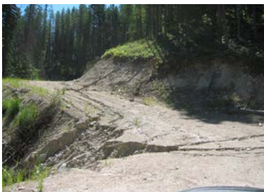
Road eroding into headwater. (Sleepy Hollow)
