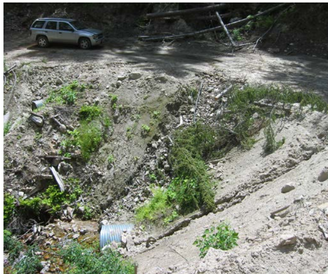
Erosion of unprotected road fill into stream. (Sleepy Hollow II)
