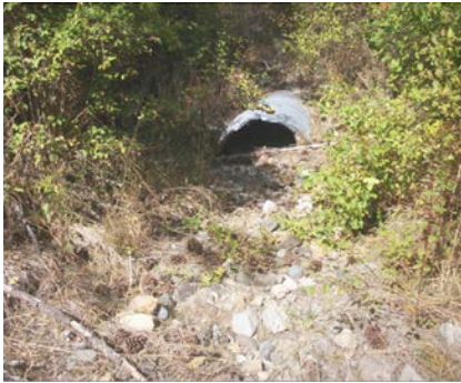
Partially plugged culvert.
