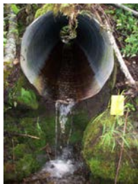
Perched culvert (barrier to fish passage)
